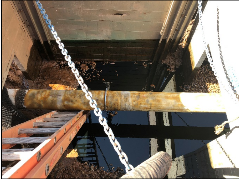
Photo 1 Oil contamination in excavation. Photo taken by SRC on August 30, 2021.
