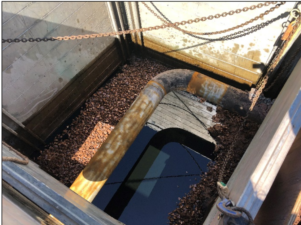
Photo 2 Oil contamination in excavation. Photo taken by SRC on August 30, 2021.
