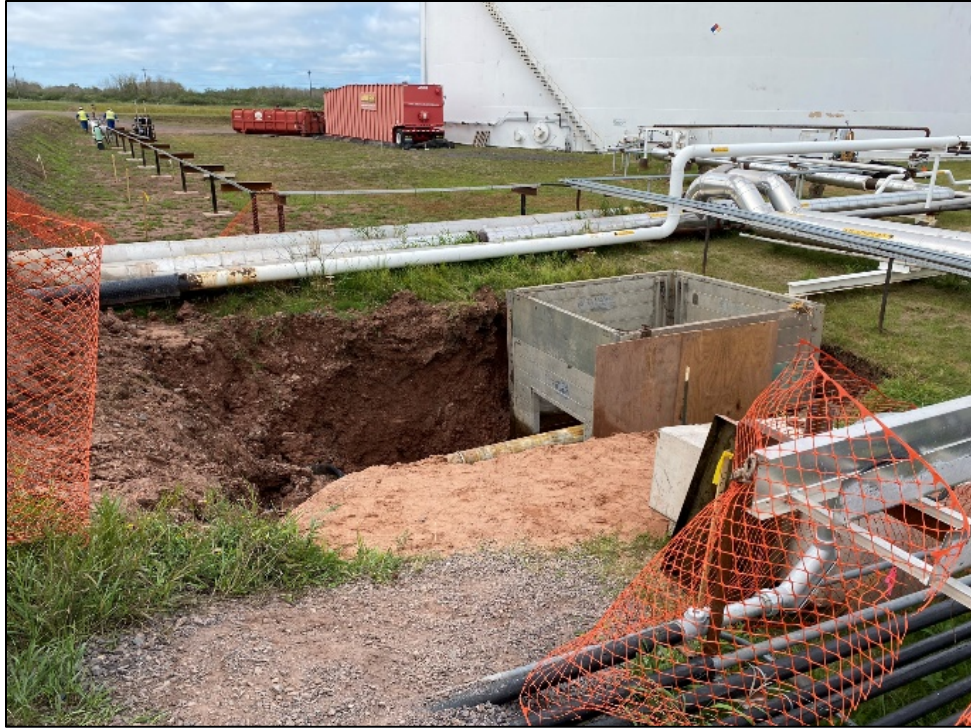
Photo 3 Excavation area before second trench box removed. Photo taken facing northwest on August 31, 2021.
