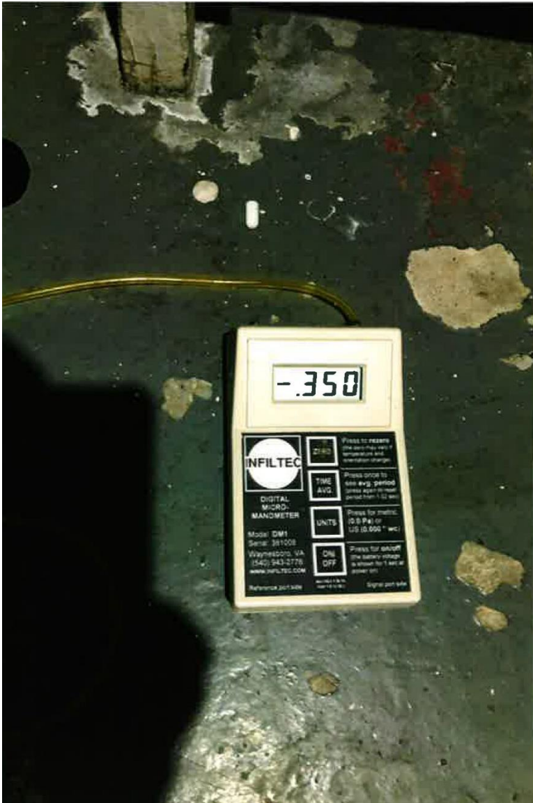
Photo 14: Sub-slab vacuum at VOP-3 following system startup.
