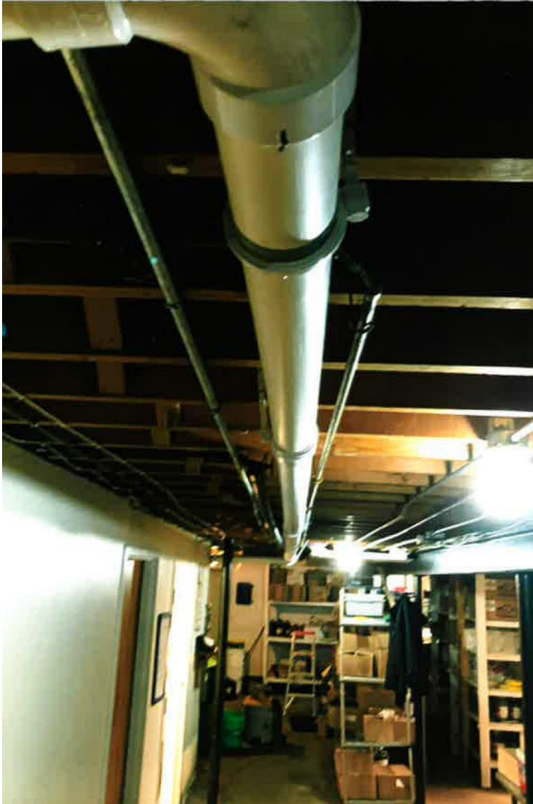
Photo 6: Piping run from Pickup Point 2.
