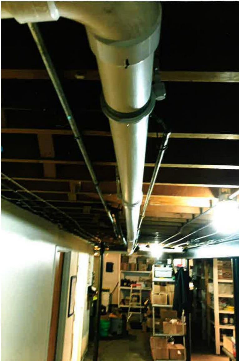
Photo 6: Piping run from Pickup Point 2.
