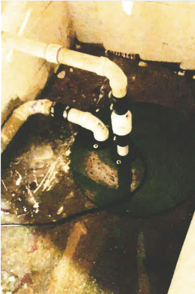
Photo 8: Sealed sump with ice machine and sump pump discharge lines.
