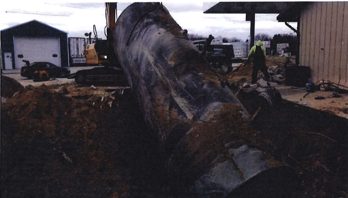
PHOTO 4 – PHOTOGRAPH OF THE 2 ND 6,000-GALLON UNLEADED GASOLINE TANK
