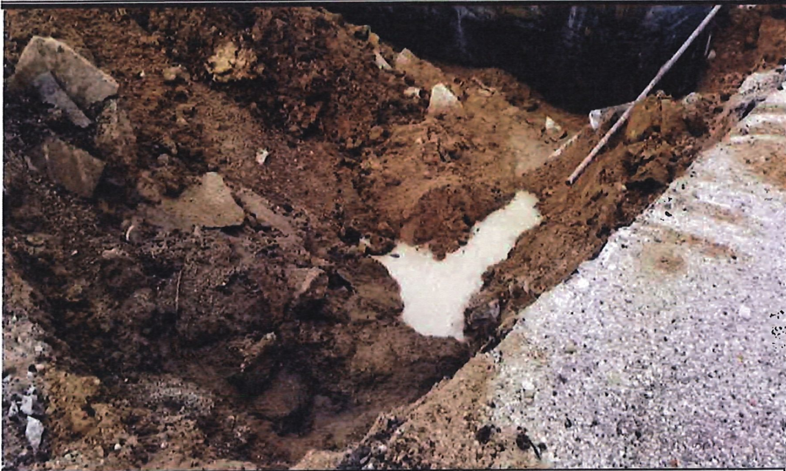
PHOTO 3 – PHOTOGRAPH OF THE SOUTHERN TANK EXCAVATION AFTER THE REMOVAL OF THE 12,000-GALLON TANK, AND THE 6,000-GALLON TANK
