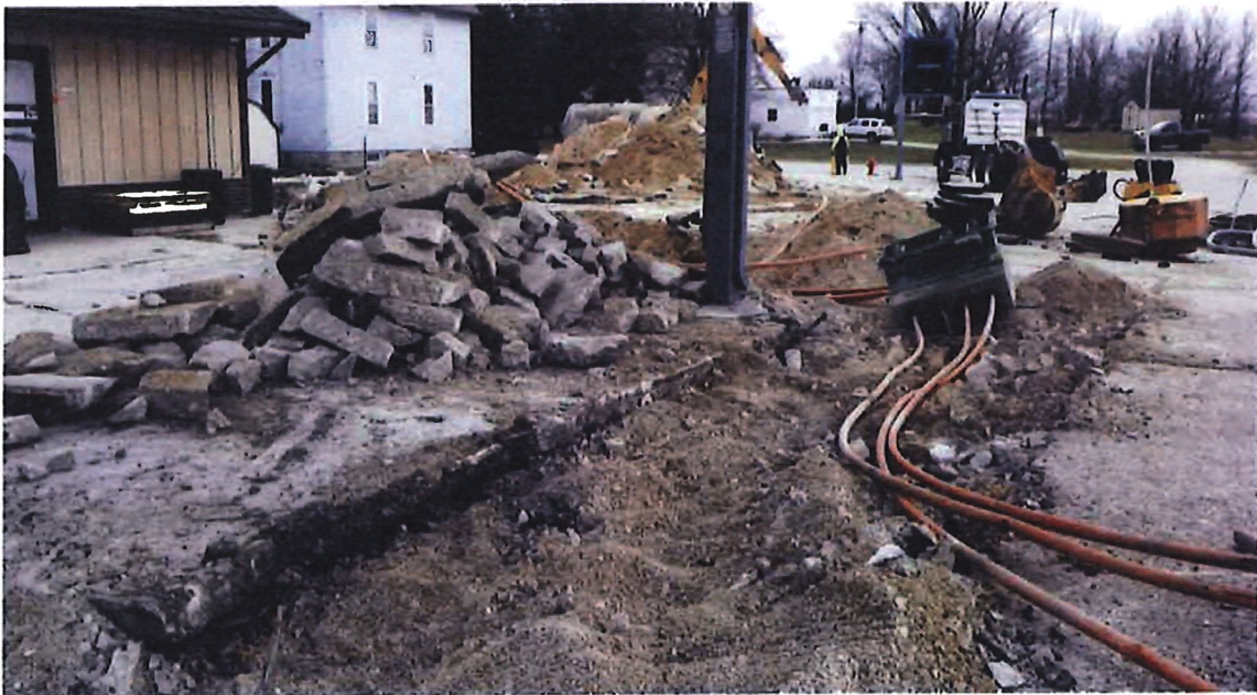
PHOTO 10 – PHOTOGRAPH OF THE DOUBLE WALL FLEX PIPE AND GASOLINE DISPENSER AREA
