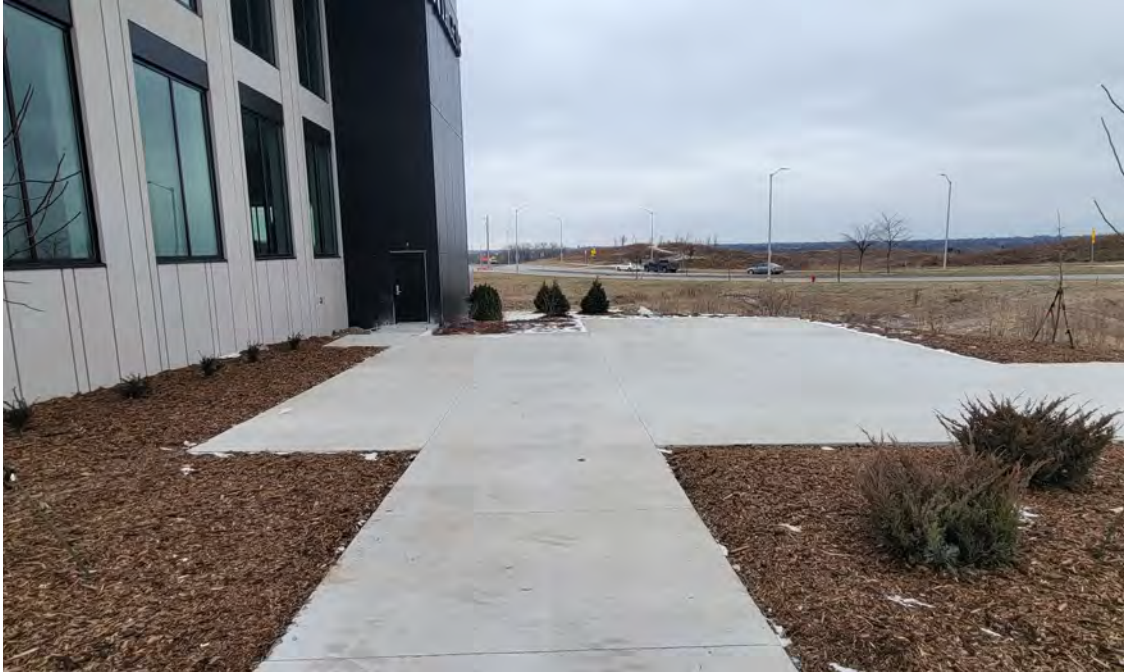
Photo 3: Construction of concrete paved patio space of Lot 3 area of the site (east side of Lot 3) with surrounding mulched landscaping (greenspace). View to north; photograph taken on December 21, 2022.
