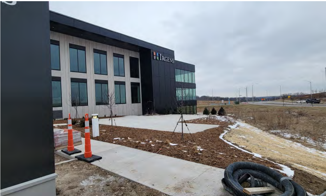
Photo 2: Construction of greenspace cap (foreground) and concrete paved sidewalk (foreground) and patio space (background) of Lot 3 area of the site (east side of Lot 3). View to northwest; photograph taken on December 21, 2022.
