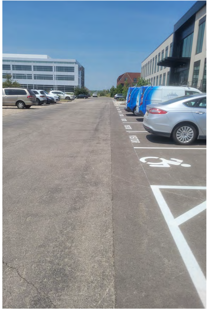
Photo 8: Asphalt paved entrance to Lot 3 and driveway along Building A. View to west; photograph taken on June 1, 2023.
