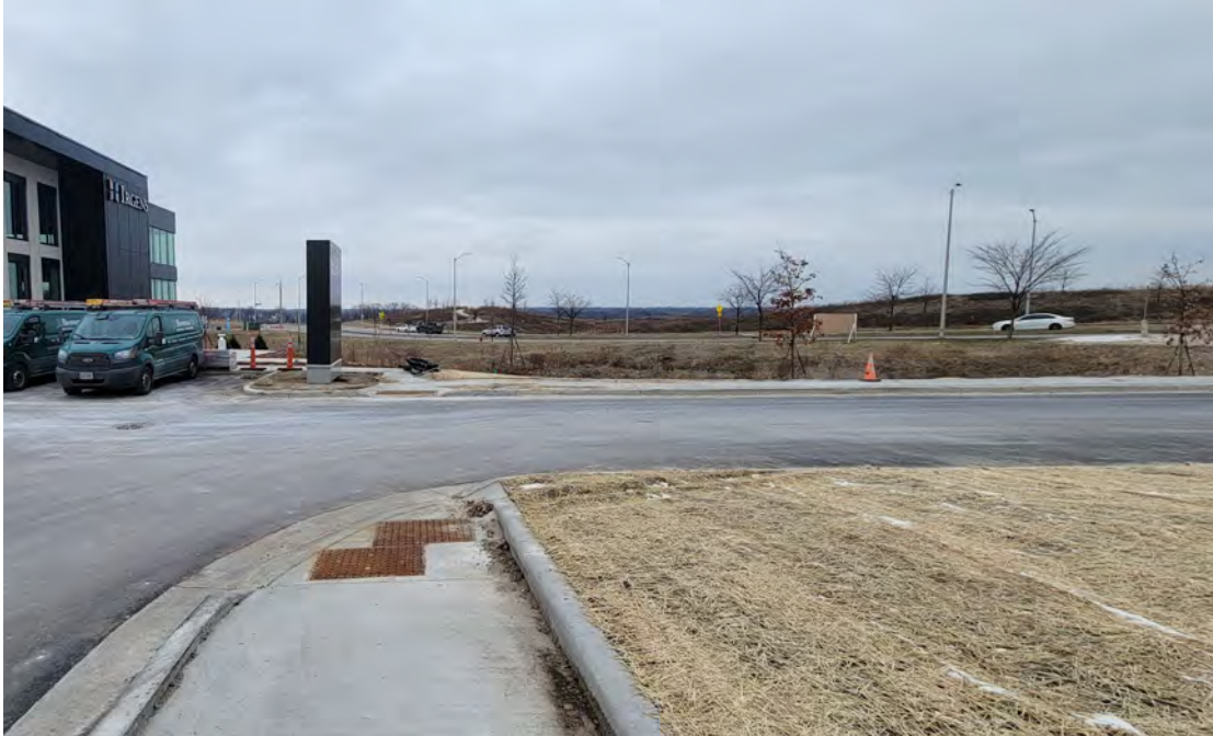
Photo 1: Construction of greenspace cap (foreground) and asphalt pavement / concrete curb and gutter cap (mid-background) within Outlot 3 area of the site. View to north; photograph taken on December 21, 2022.
