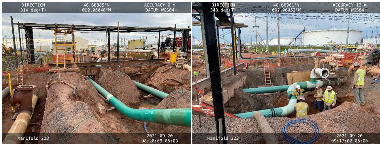
Photo 7: Middle portion of the final project excavation. The Line 1 PCV infrastructure is beyond the black equipment rack. Photo taken facing northwest on September 20, 2021.
