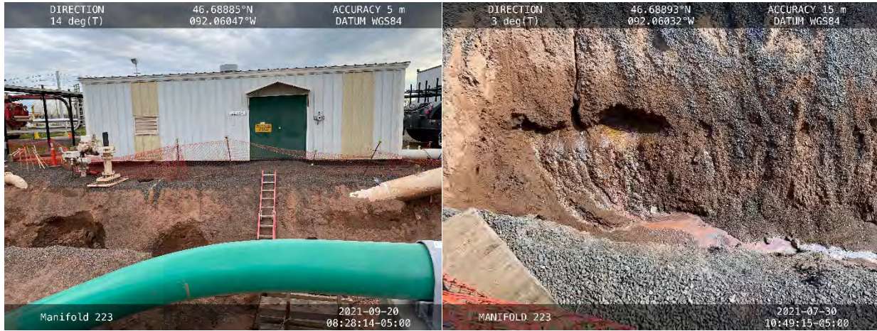
Photo 5: Line 2 PCV building and final project excavation sidewall. Photo taken facing north on September 20, 2021.
