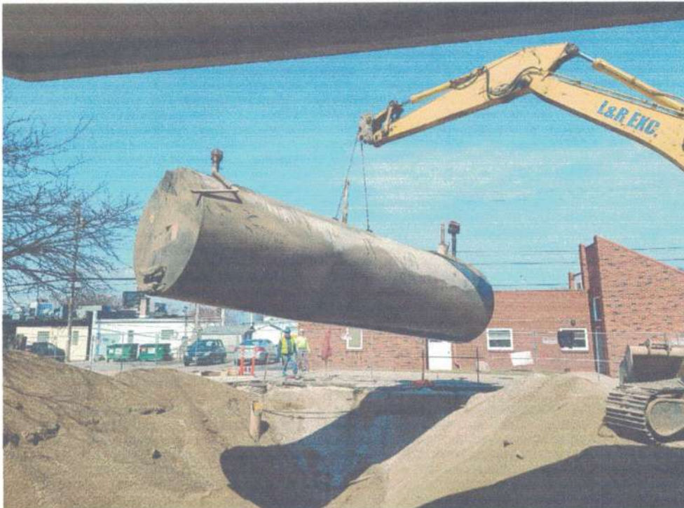
PHOTOGRAPH OF THE SECOND 12,000-GALLON UST JUST AFTER REMOVAL FROM THE EXCAVATION
