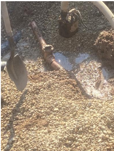
Location of initial break and upwelling. No municipal water from this area reached the catch basin.
