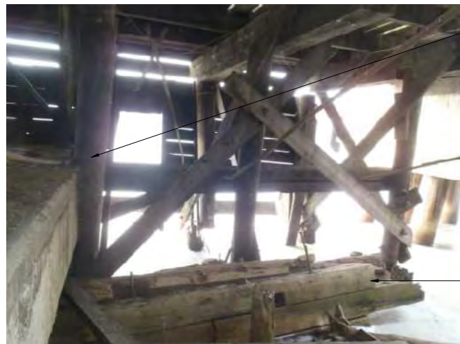
TIMBER PILE ENCASED IN CONCRETE TO BE CUT AND REMOVED AT UPPER FACE OF CONCRETE
