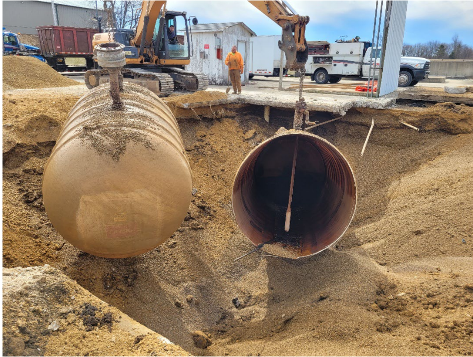
PHOTOGRAPH OF THE THIRD UST. TANK BROKE IN HALF BUT NOT PRODUCT WAS SPILLED
