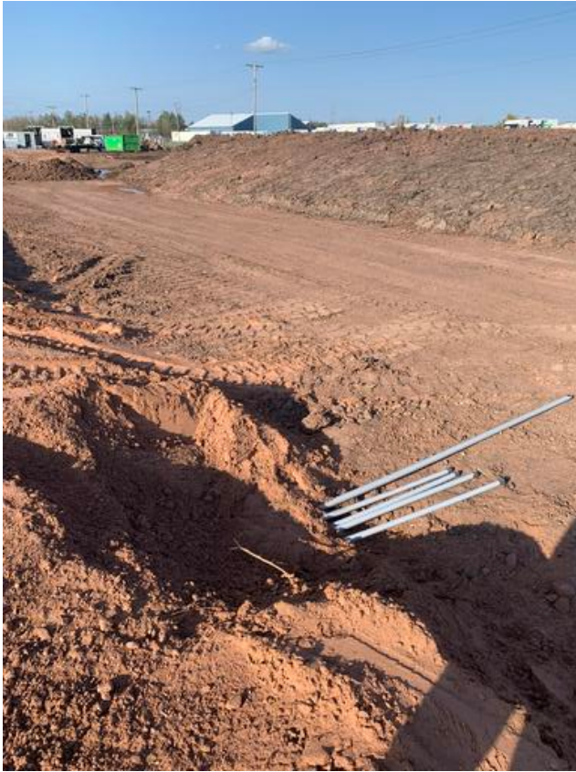
Conduit Extensions @ East Van Lot
