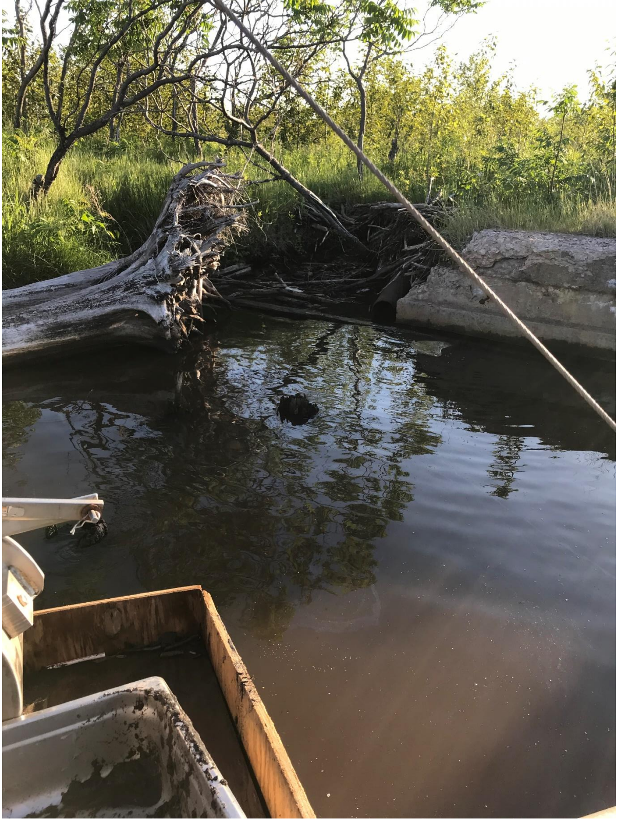
Pipe (possible outfall) next to concrete at the head of the Amoco Barge Slip, Superior Wi. Viewing south. Taken July 2, 2022, by Joe Graham.
