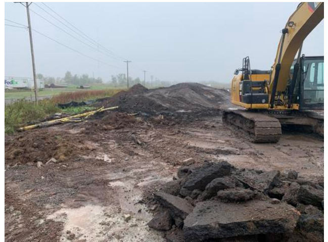
Pond berm & debris
