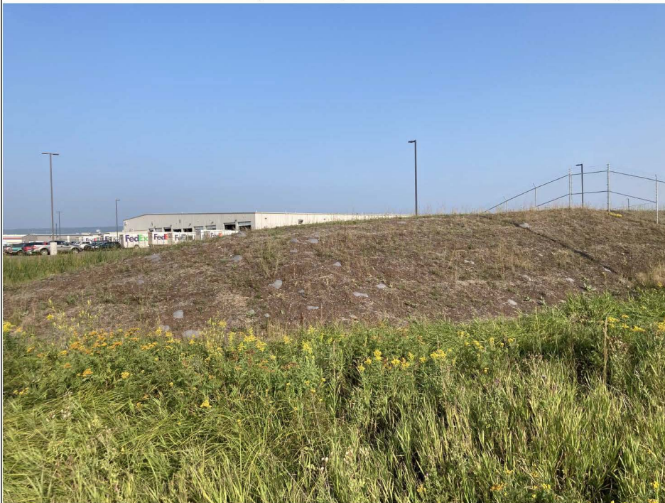
Title: South end of berm, viewing northwest, note little to no vegetation and numerous exposures of cap liner material.
