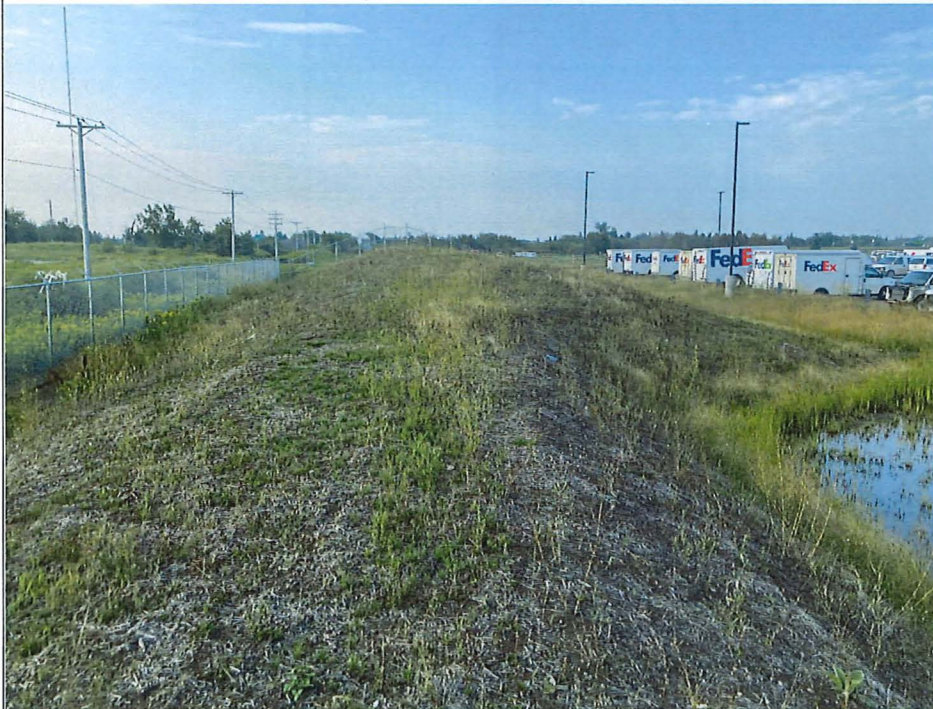
Title: Berm viewing south, storm water detention pond on right. Note scarce vegetation.
