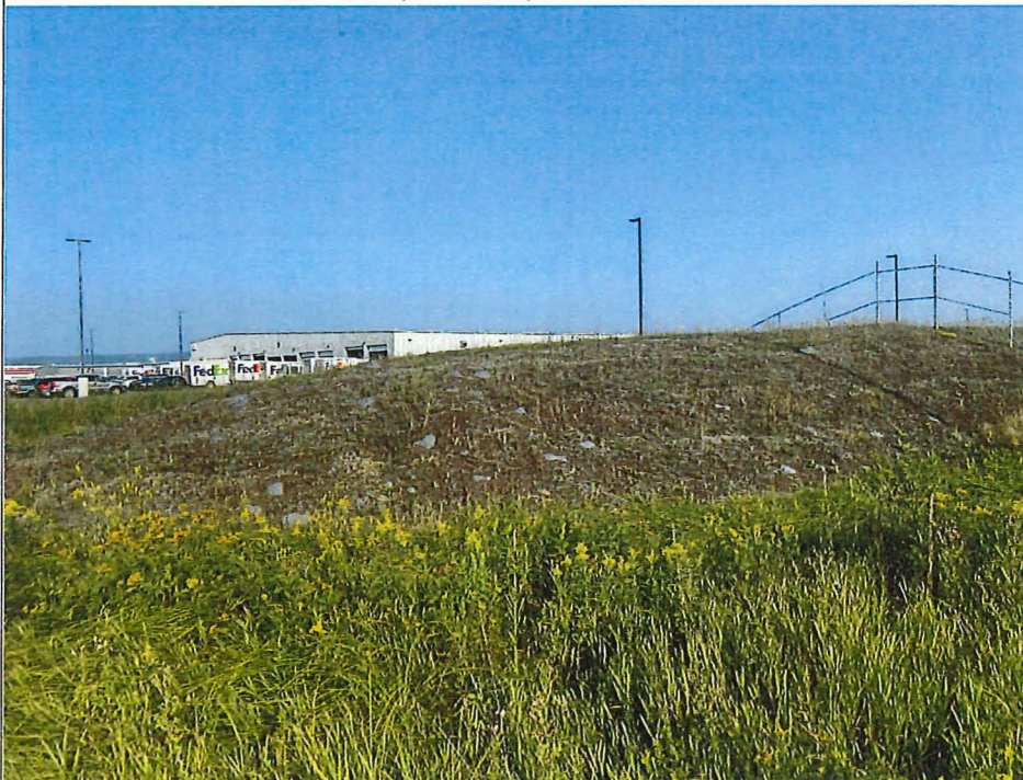
Title: South end of berm, viewing northwest, note little to no vegetation and numerous exposures of cap liner material.
