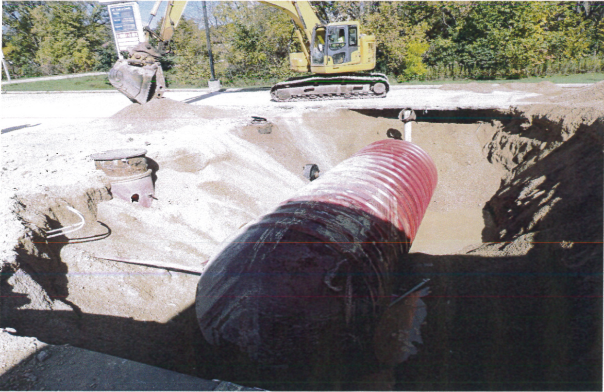
Photo 4 – Southern UST exposed in basin
