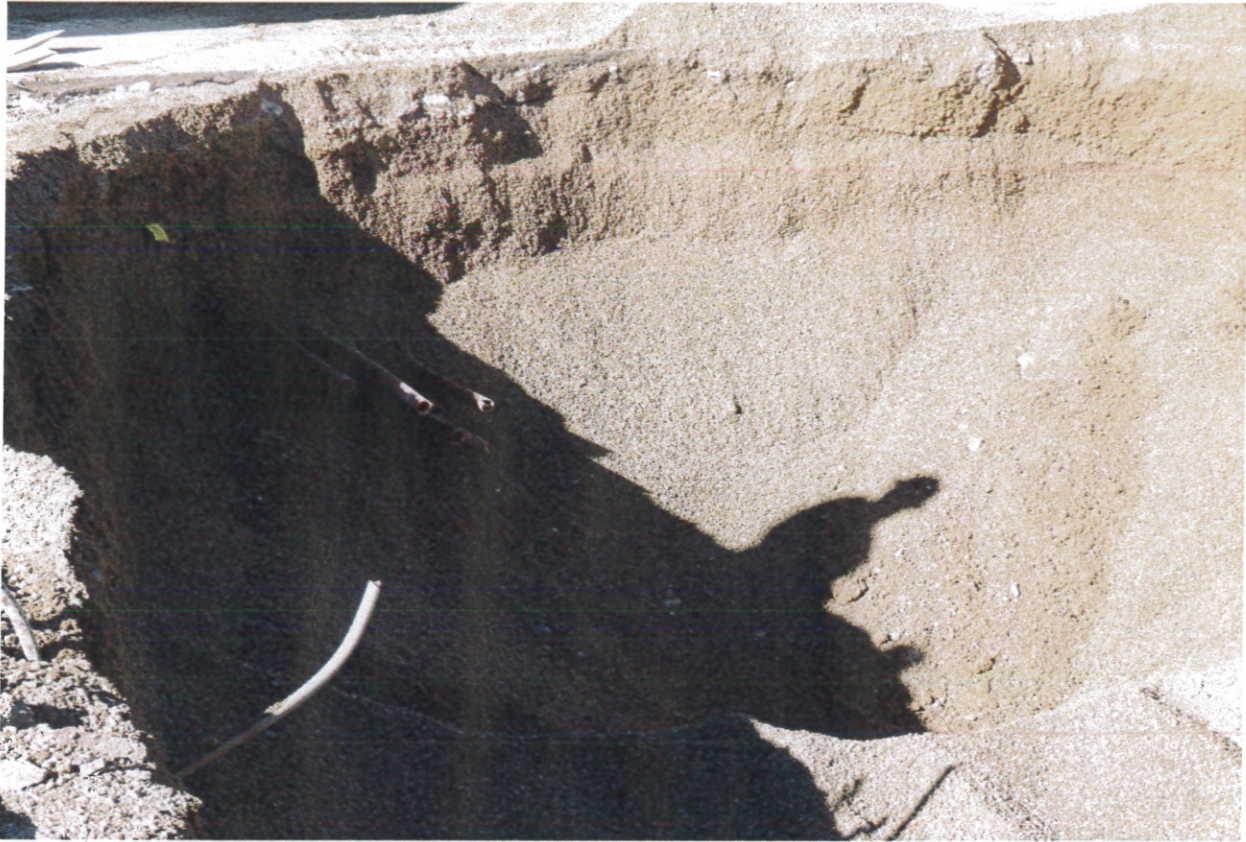
Photo 11 – View of distribution piping heading out of northwest corner of UST basin to dispensers
