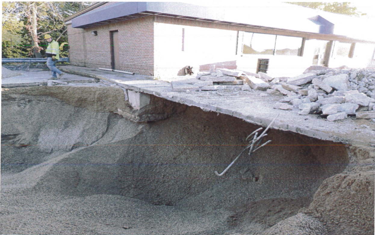
Photo 12 – View of pea stone backfilling along southwest wall of basin – no native soil encountered.
