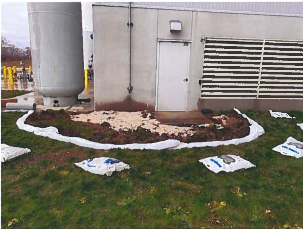
Mid-Project: Hydrophobic absorbent booms placed inside trench surrounding perimeter of release area.
