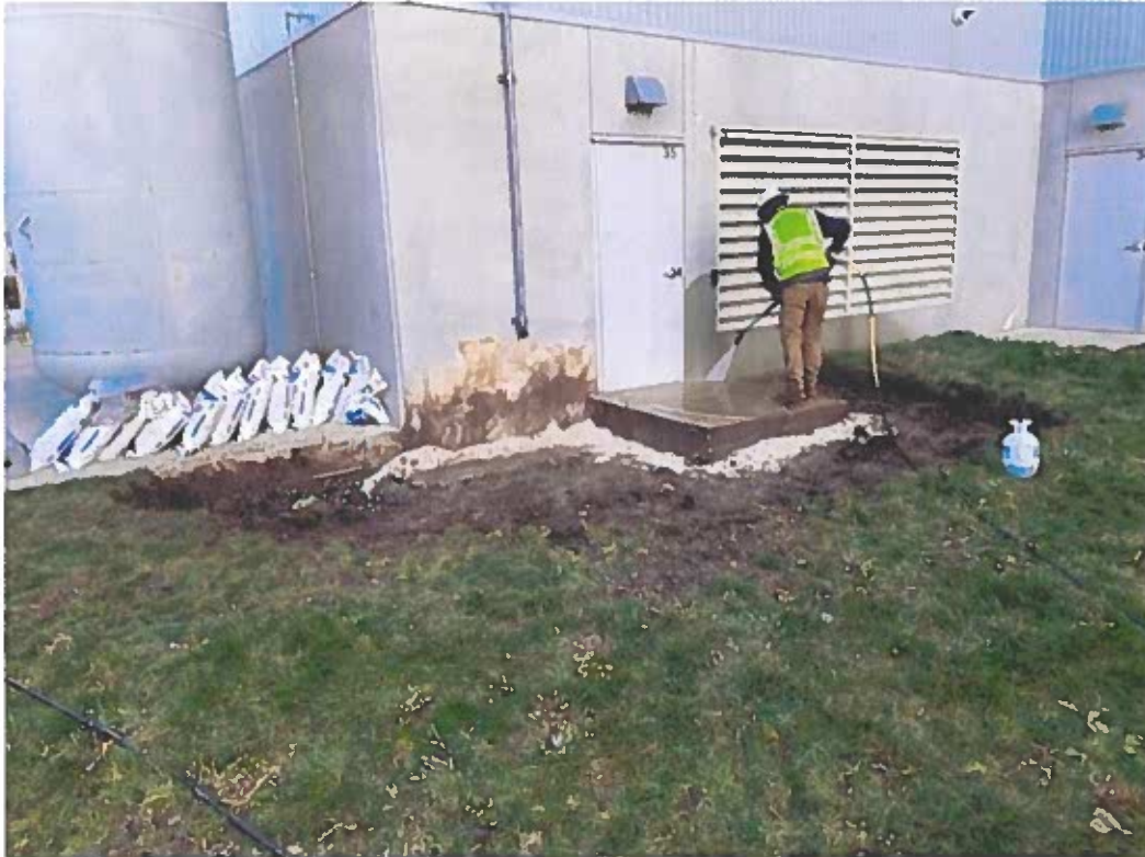
Mid-Project: Pressure washing the impacted wall and concrete slab following the detergent application.
