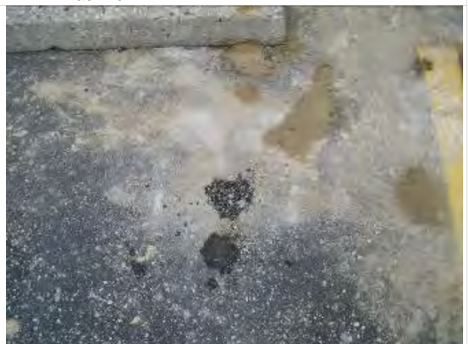
6. A view of boring B-1 patched with asphalt.
