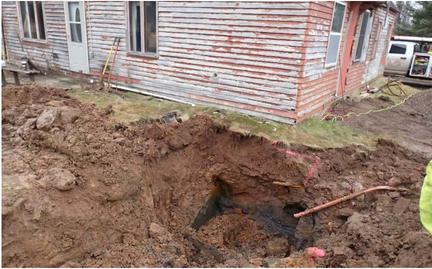
Stained soil underneath removed 550-gallon tank, facing southwest.
