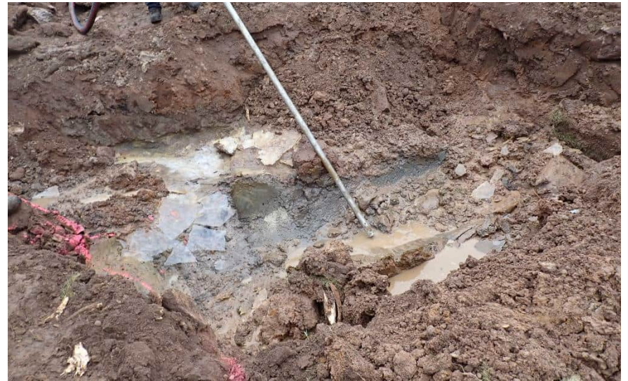
Stained soils underneath removed 750-gallon tank as observed during the pumping of liquid from the basin
