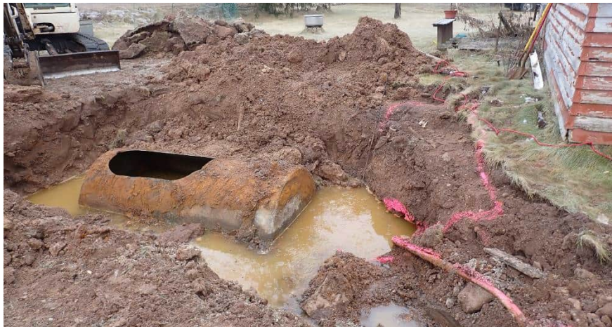
Excavation area, facing south. Liquid in and around the tank was pumped or off-site disposal
