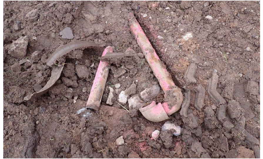
Piping related to former dispensers.
