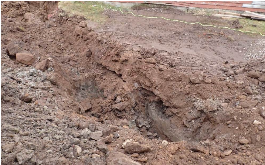
Stained soils underneath former dispenser area.
