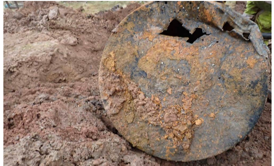
Deteriorated 550-gallon tank, removed.
