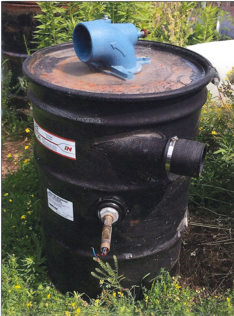
PHOTO OF KNOCKOUT TANK AND HIGH LEVEL SWITCH PROVIDED BY SCS ENGINEERS
