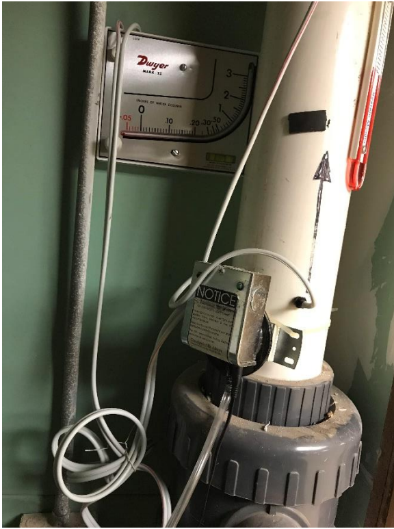
Photo 5: Sub-slab depressurization mitigation system alarm system and vacuum gauge. Alarm not functioning 01/07/2019.
