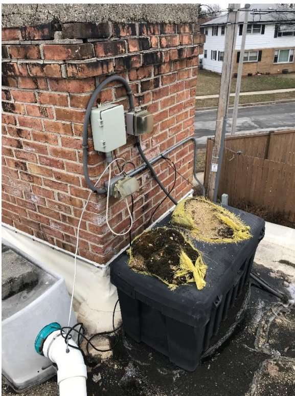
Photo 10: Sub-slab depressurization mitigation system and drain tile ventilation system electrical connections 01/17/2019
