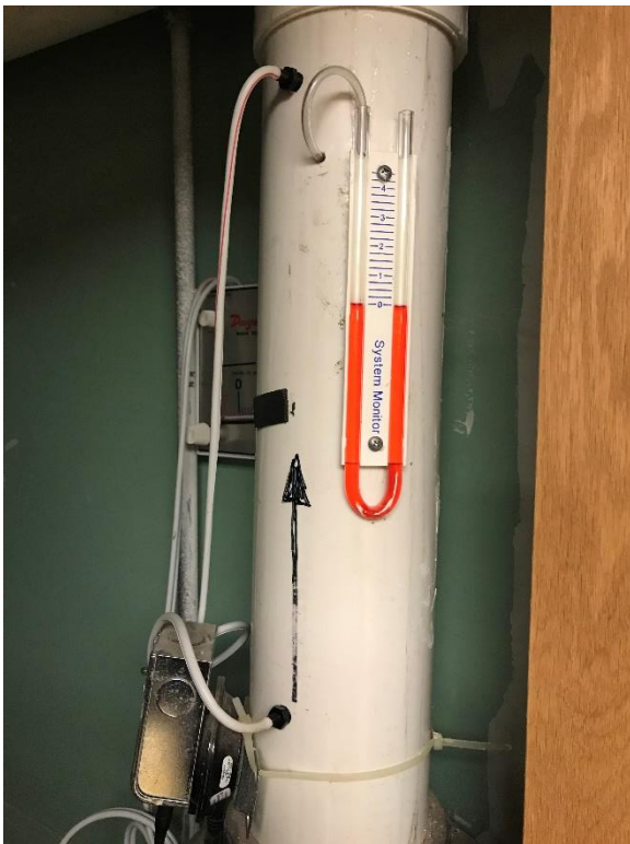
Photo 4: Sub-slab depressurization mitigation system manometer reading zero vacuum 01/07/2019
