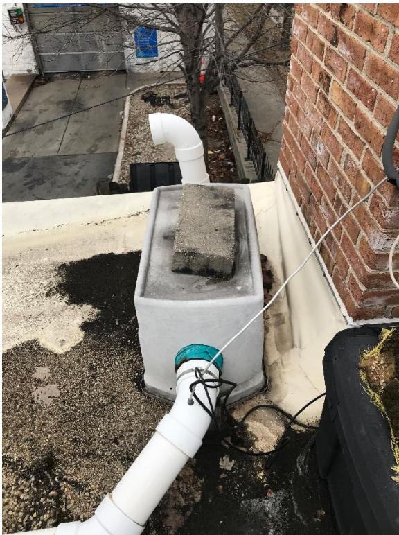
Photo 8: Drain tile ventilation system blower box 01/17/2019
