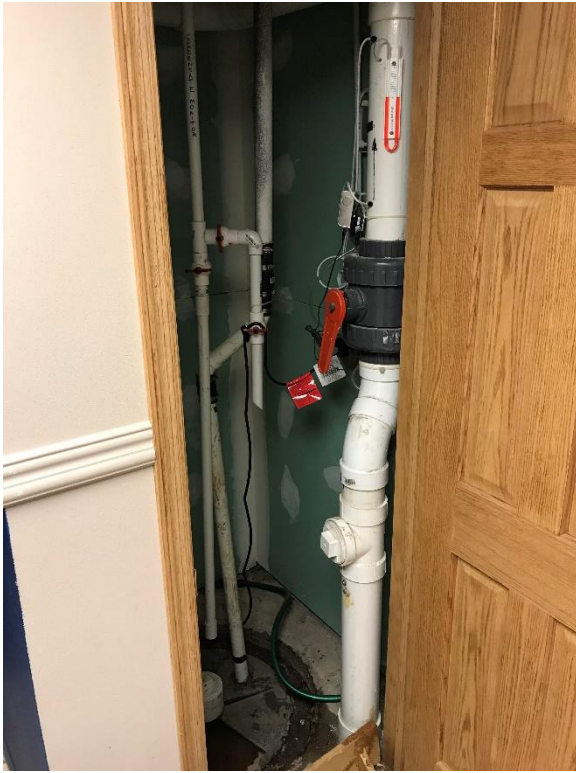
Photo 3: Sump 1 with sub-slab depressurization mitigation system vacuum pipe and manometer 01/07/2019
