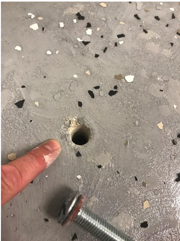
Photo 12: RA Environmental sub-slab vacuum observation point and plug, typical 08/06/2019
