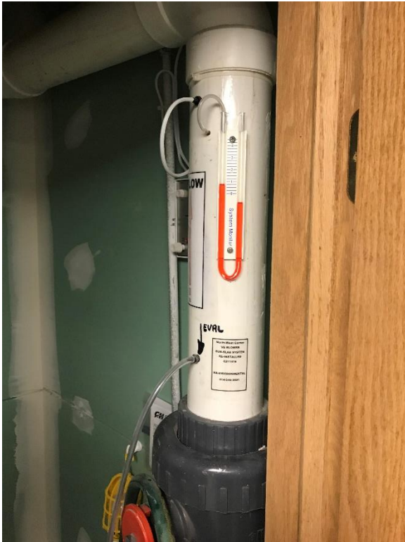
Photo 21: Manometer on sub-slab depressurization mitigation system piping after drain tile ventilation system and sub-slab depressurization mitigation system turned back on 08/14/2019
