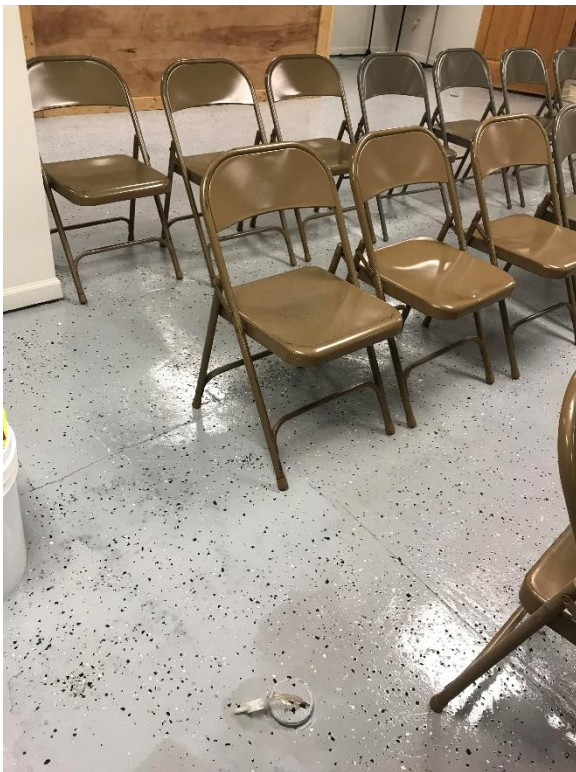
Photo 14: Sub-slab depressurization mitigation system cleanout lid fitted with tubing for sub-slab pressure field extension testing, typical 08/06/2019
