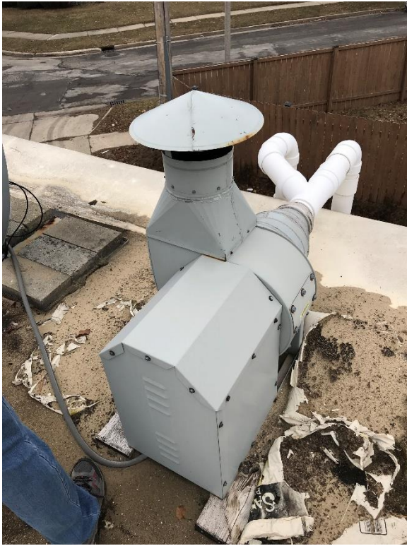
Photo 7: Sub-slab depressurization mitigation system blower on Grace roof, not operating 01/17/2019
