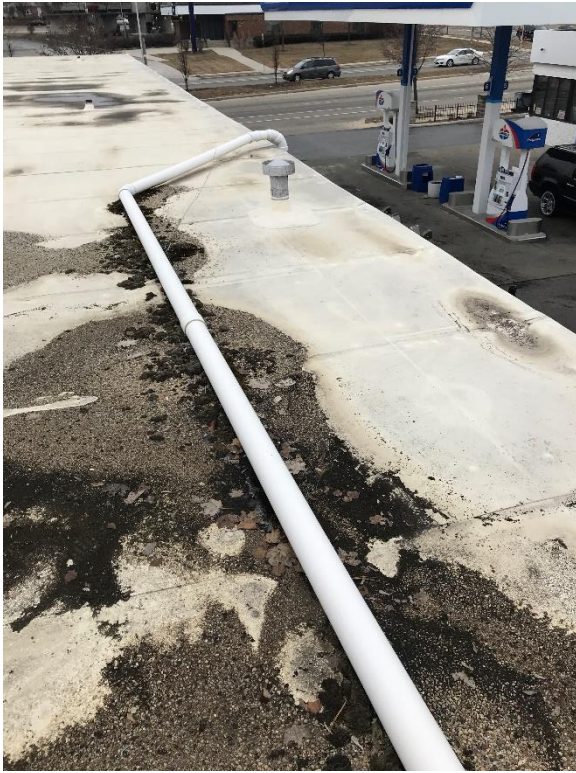
Photo 11: Drain tile ventilation system vacuum piping 01/17/2019
