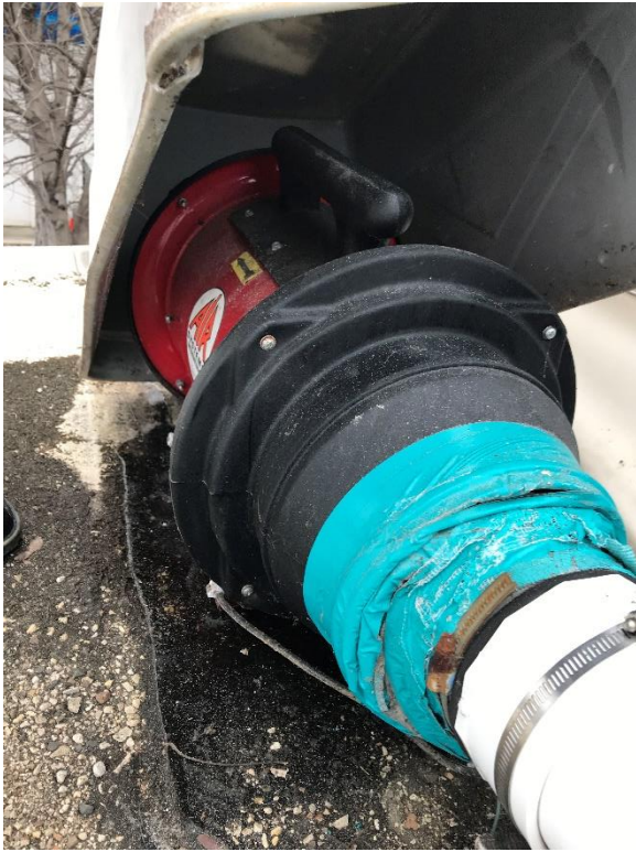
Photo 9: Drain tile ventilation system blower not operating 01/17/2019
