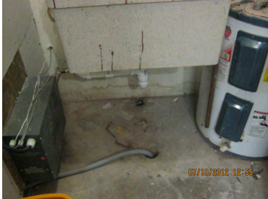
Photo 6: View of the floor drain observed in the eastern-most building on the Lesperance parcel.
