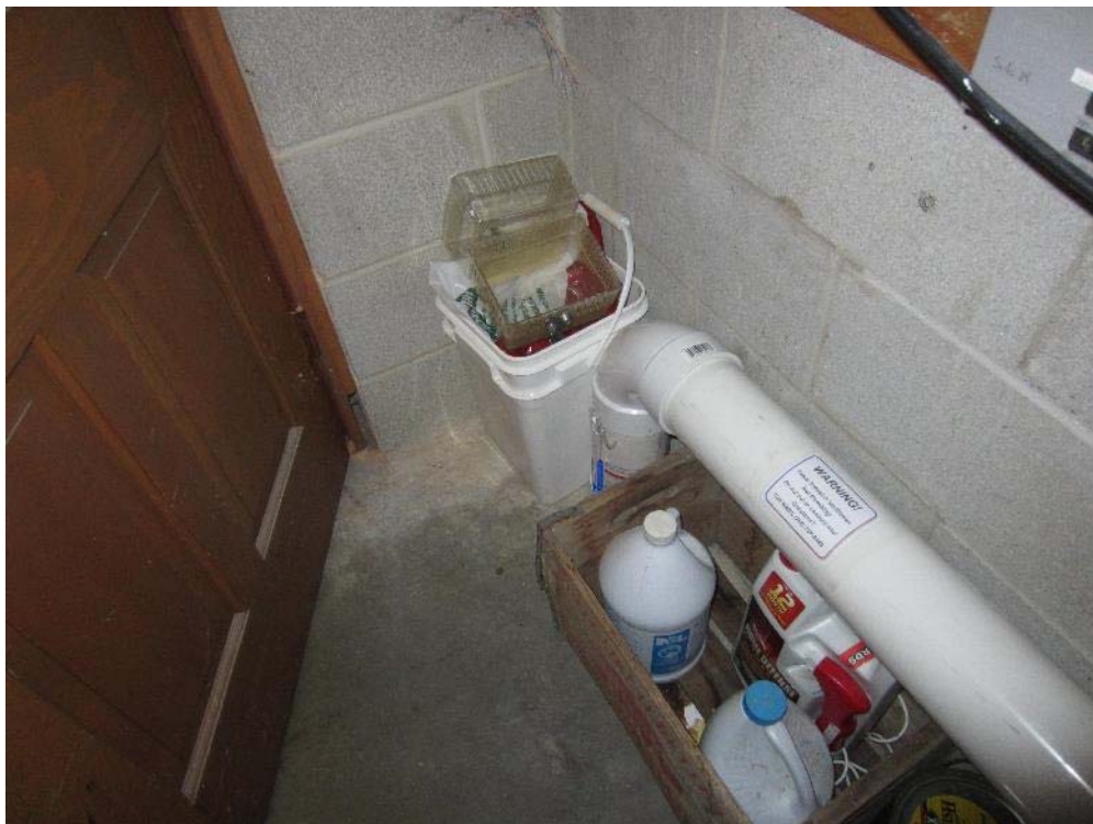
Photo 6: Southwest utility room extraction point and manometer
