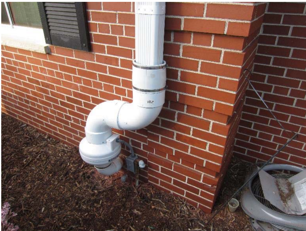
Photo 8: Southwest system fan
