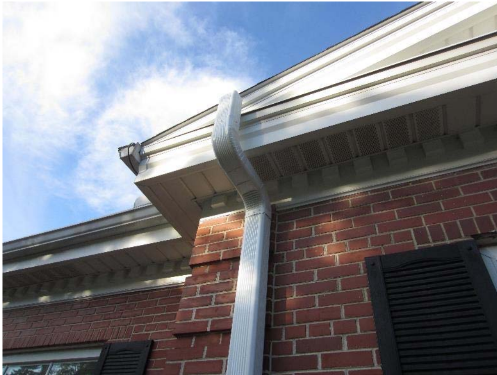
Photo 5: Northwest system exhaust location
