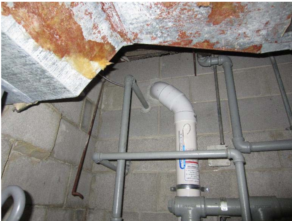
Photo 2: Northwest furnace room wall penetration and manometer
