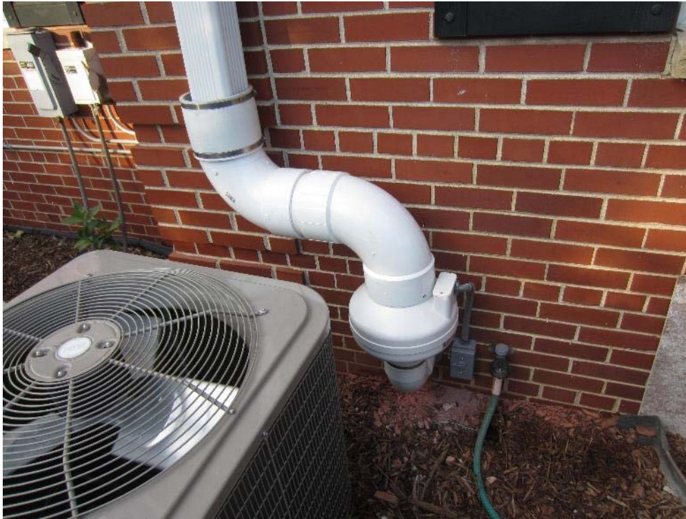
Photo 3: Northwest system fan
