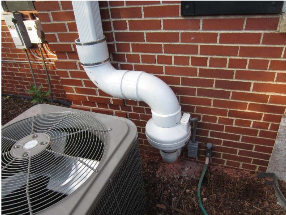
Photo 3: Northwest system fan
