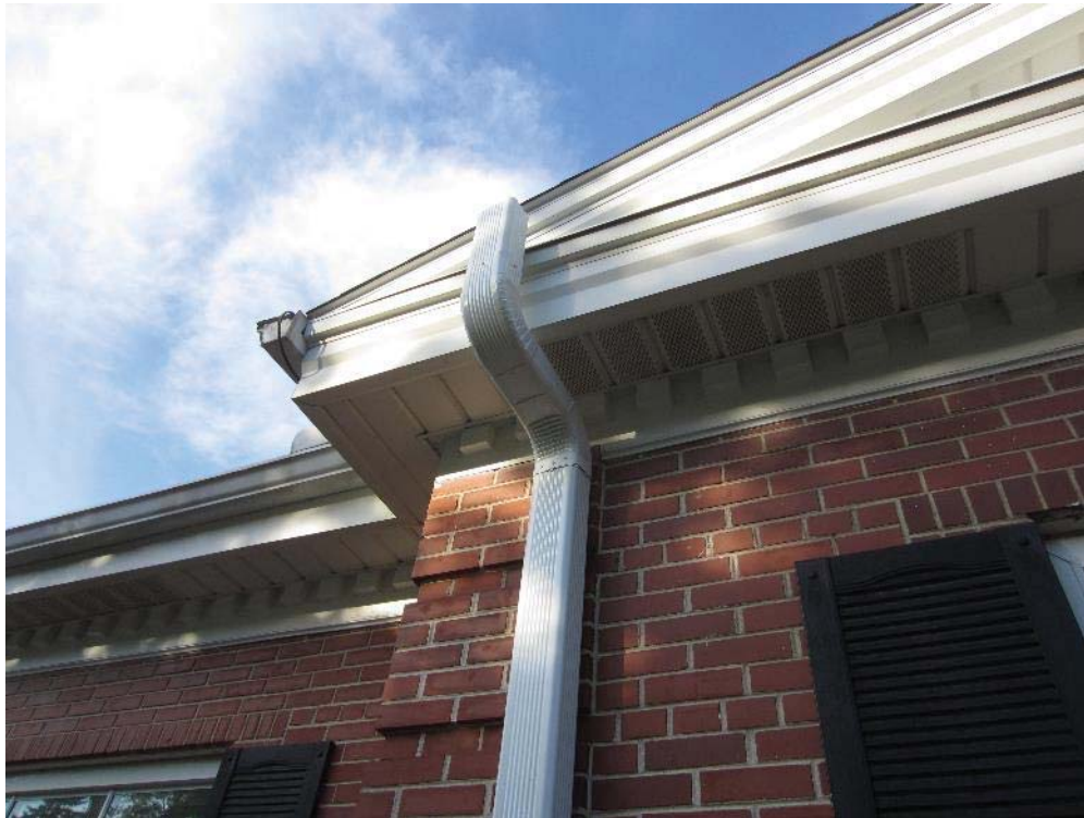
Photo 5: Northwest system exhaust location
