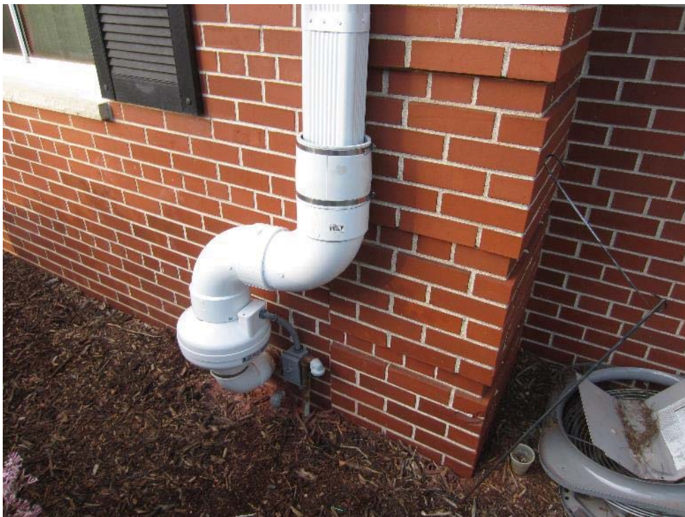
Photo 8: Southwest system fan
