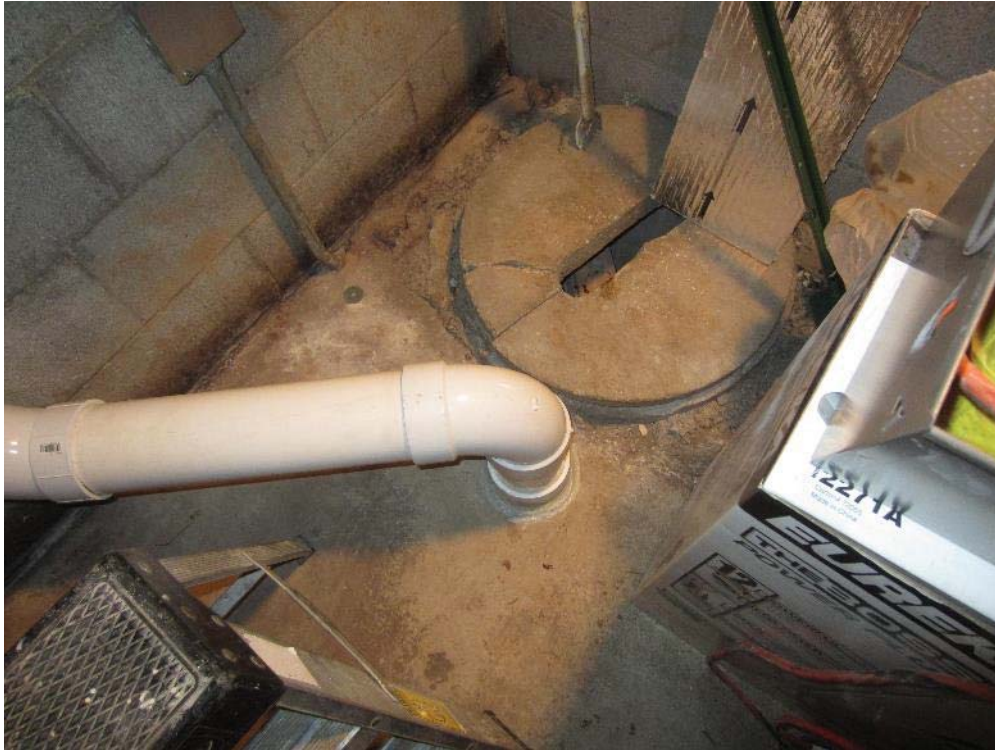
Photo 1: Northwest furnace room extraction point
