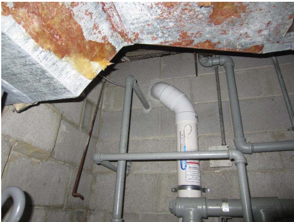
Photo 2: Northwest furnace room wall penetration and manometer
