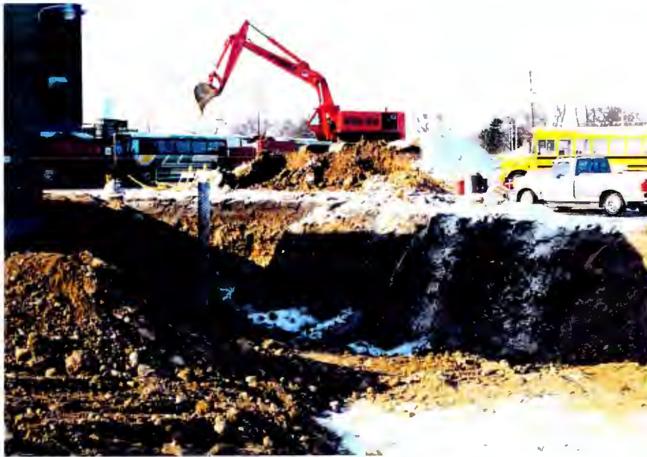
Excavation looking southwest, with clean overburden soil pile west of the excavation.
