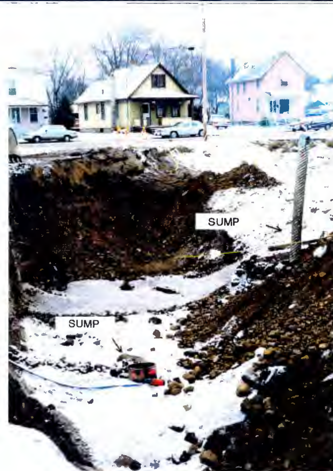
Excavation looking north -- eastern portion partially backfilled, with pump and sump in the foreground.
