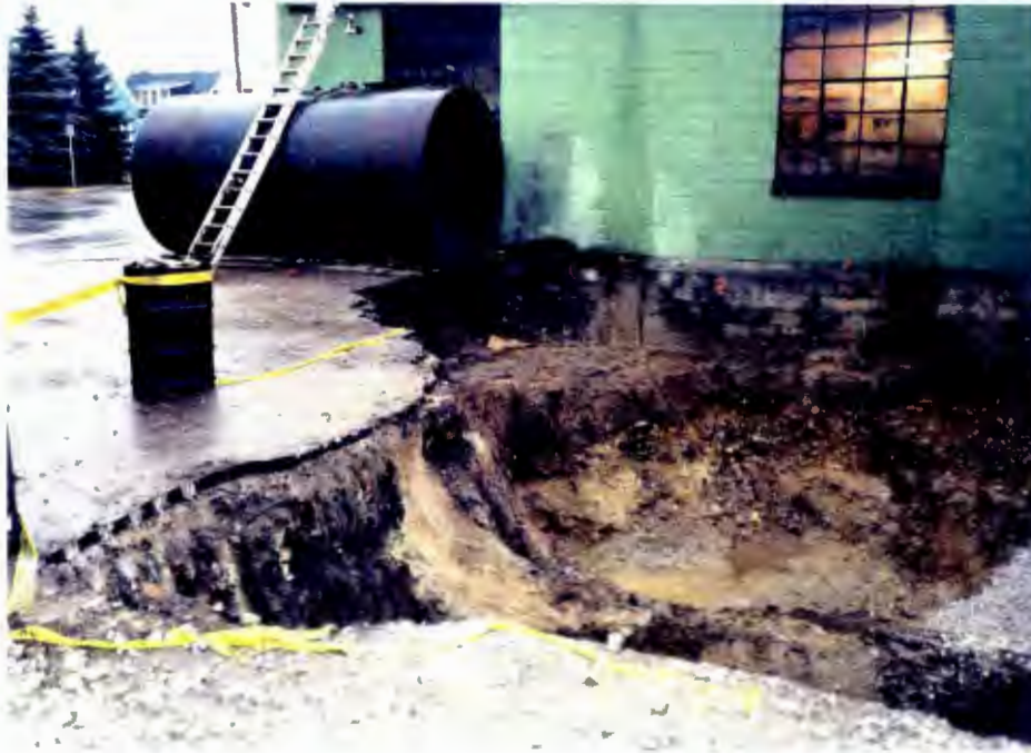
Northern end of excavation showing tank used to temporarily store excavation water.
