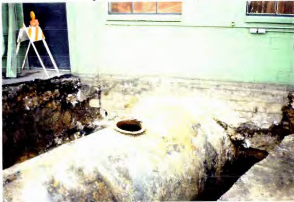
6000 gallon diesel tank lodged under building.
