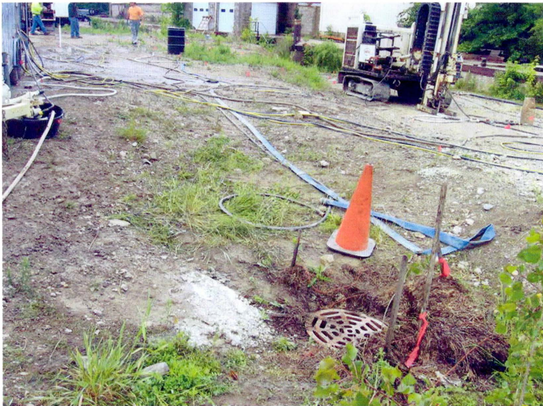
Photo 4 – Injecting into direct push borings at lateral L4 and L5 treatment areas. Storm sewer in foreground.
