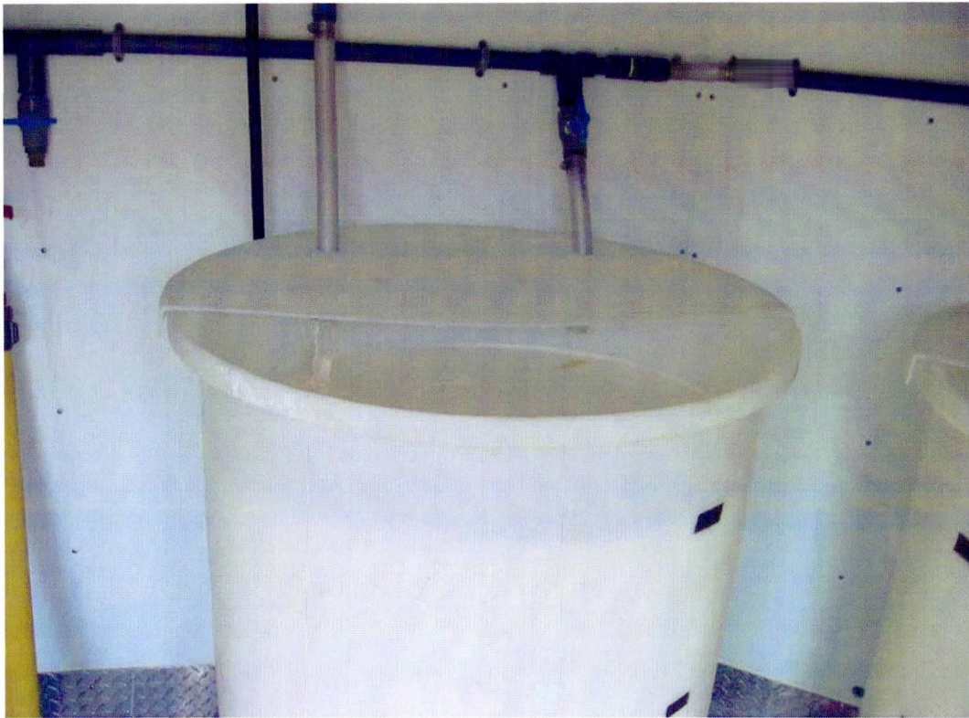
Photo 3 – Mixing tank inside trailer where concentrated EOS is mixed with water.
