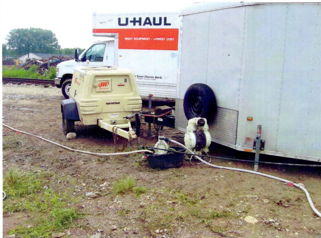
Photo 2 – Pumps used to pump concentrated EOS from tanker (or totes) into trailer for mixing.
