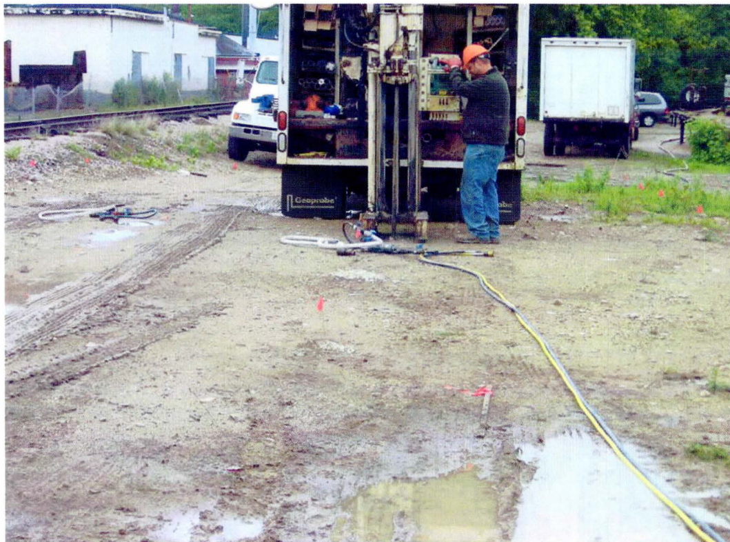
Photo 6 – Injecting into direct push boring at treatment area L4 showing hose from mixing trailer. Injection is controlled at well head using valves and flow meter shown above.
