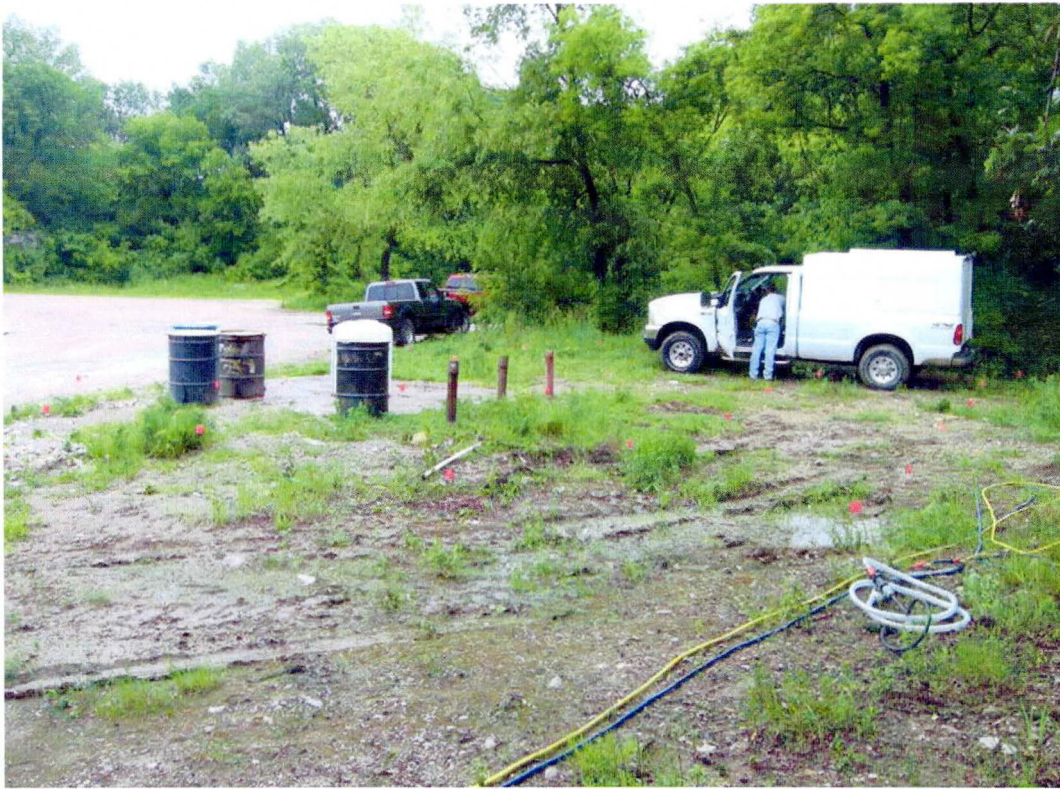
Photo 9 – Advancing direct push boring and injecting EOS at lateral L1 treatment area near MW-04 well nest.
