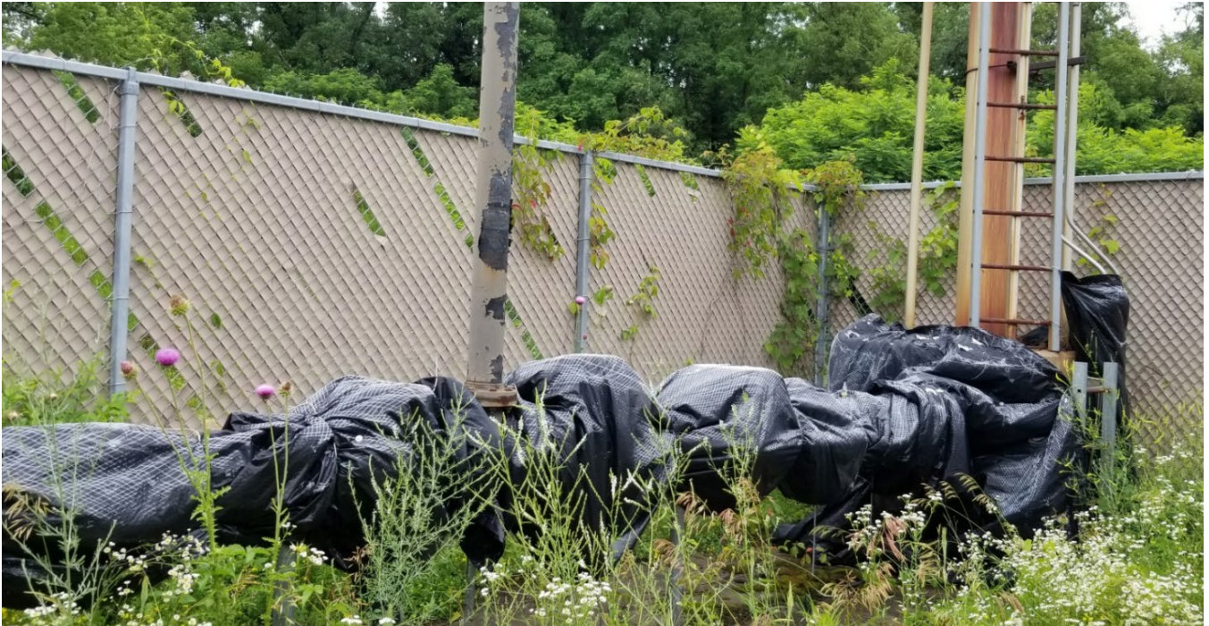
Old stack system with degrading and insufficient insulation.
