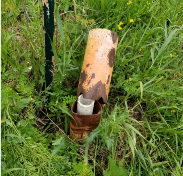
Broken steel casings on wells
