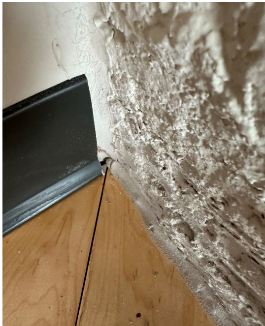
Photo 30 – Gap/hole between baseboard and wall
