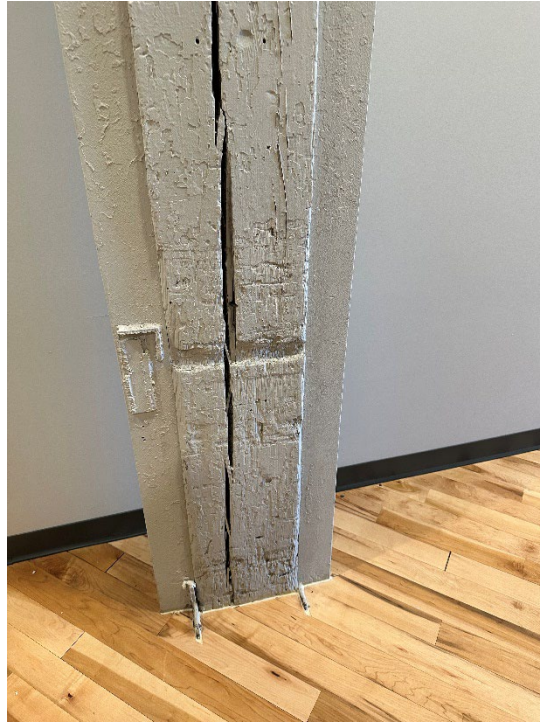
Photo 19 - Wood post is split and is not sealed all around
