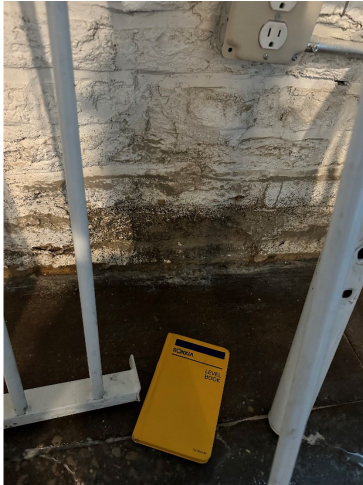
Photo 9 – Deterioration along masonry wall
