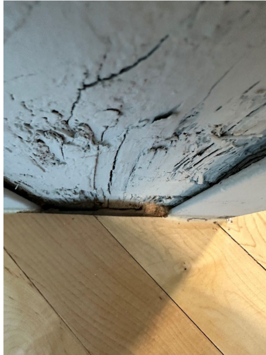
Photo 21 - Gap between wood post and floor. Wood is split and porous
