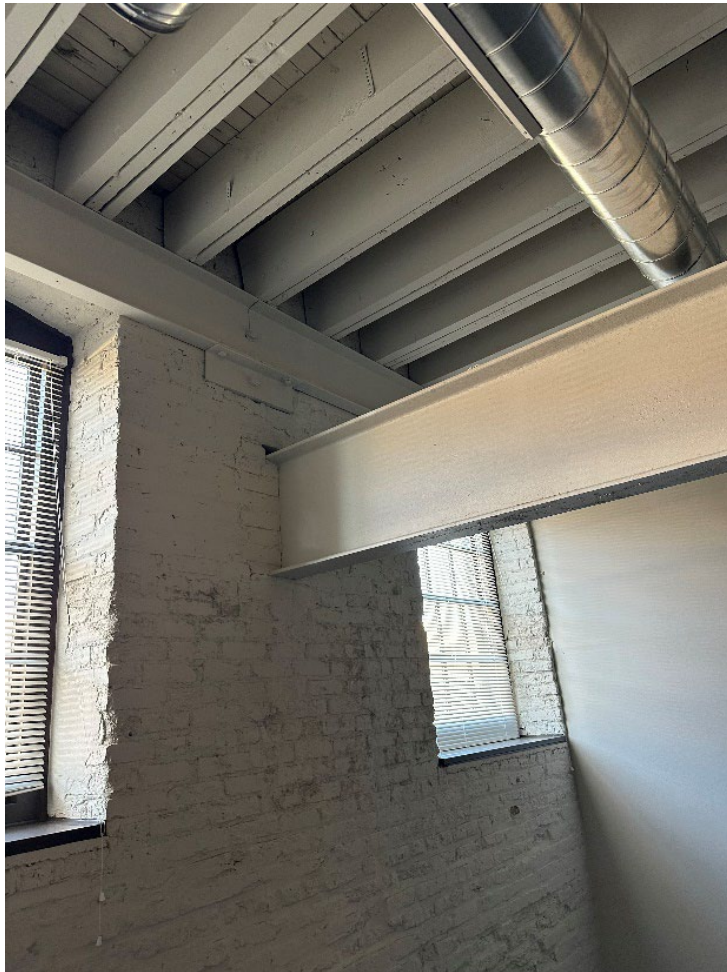
Photo 8 – Gap above I-beam and masonry wall
