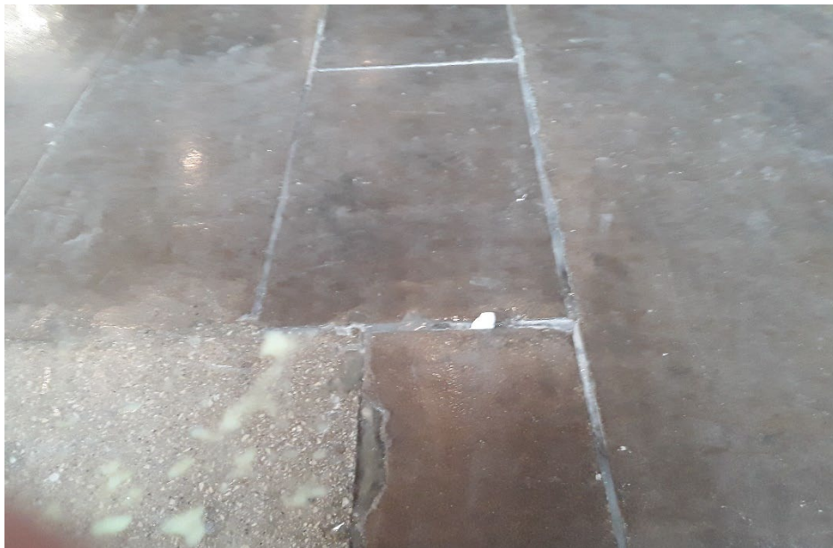
Photo 37 – Example of additional temporary fixes in the flooring
