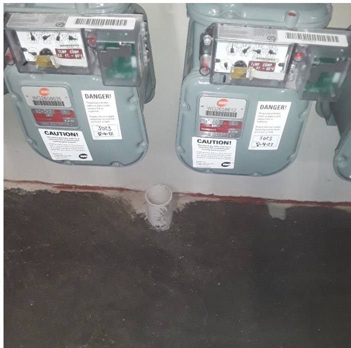
Photo 41 – Missing Pipe Cap that needs to be capped
