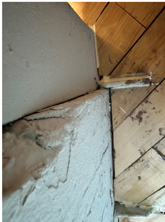
Photo 20 - Posts are not sealed all the way around and the wood beams are very porous
