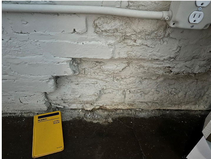
Photo 6 - Deterioration along masonry wall and small gaps between the slab and wall
