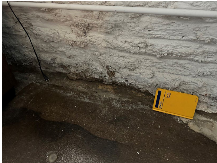
Photo 5 - Deterioration of masonry wall
