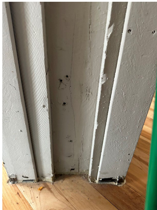
Photo 22 - Gaps between floor and the masonry wall. The wood post is porous and not sealed.
