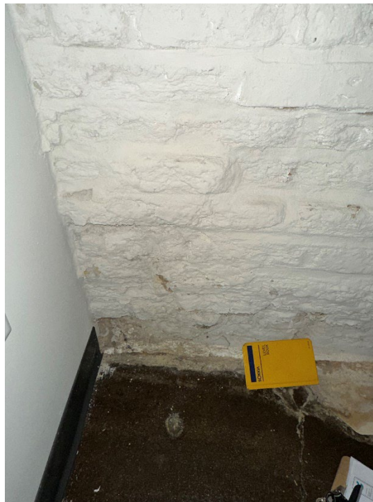
Photo 7 – Deterioration along masonry wall and small gaps between the slab and wall
