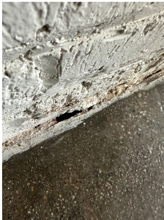
Photo 14 - Gaps between all along the masonry wall and slab
