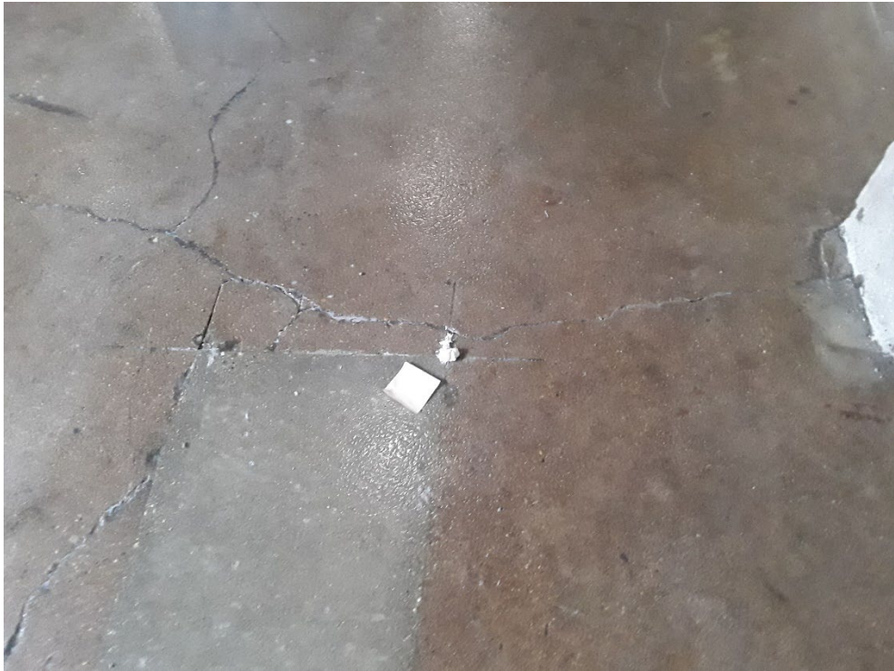
Photo 36 – Leaking Saw Cut near SDDS Pipe End
