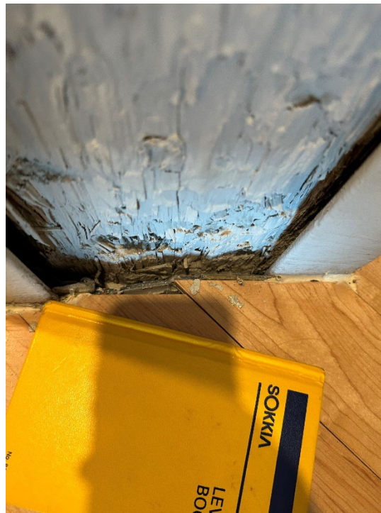
Photo 25 – Gaps between wood post and floor, post is not sealed all the way around
