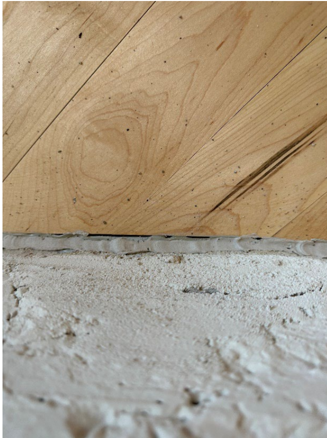
Photo 23 – Small gaps between floor and masonry wall
