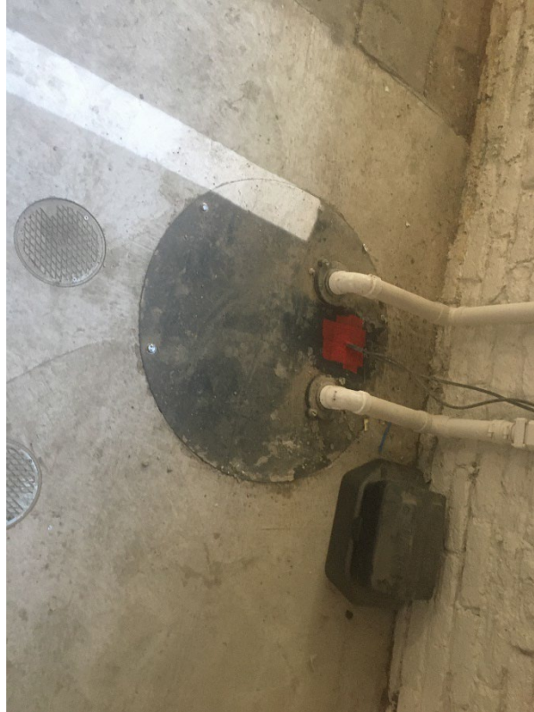
Photo 37 – Sump crock needs to be sealed permanently
