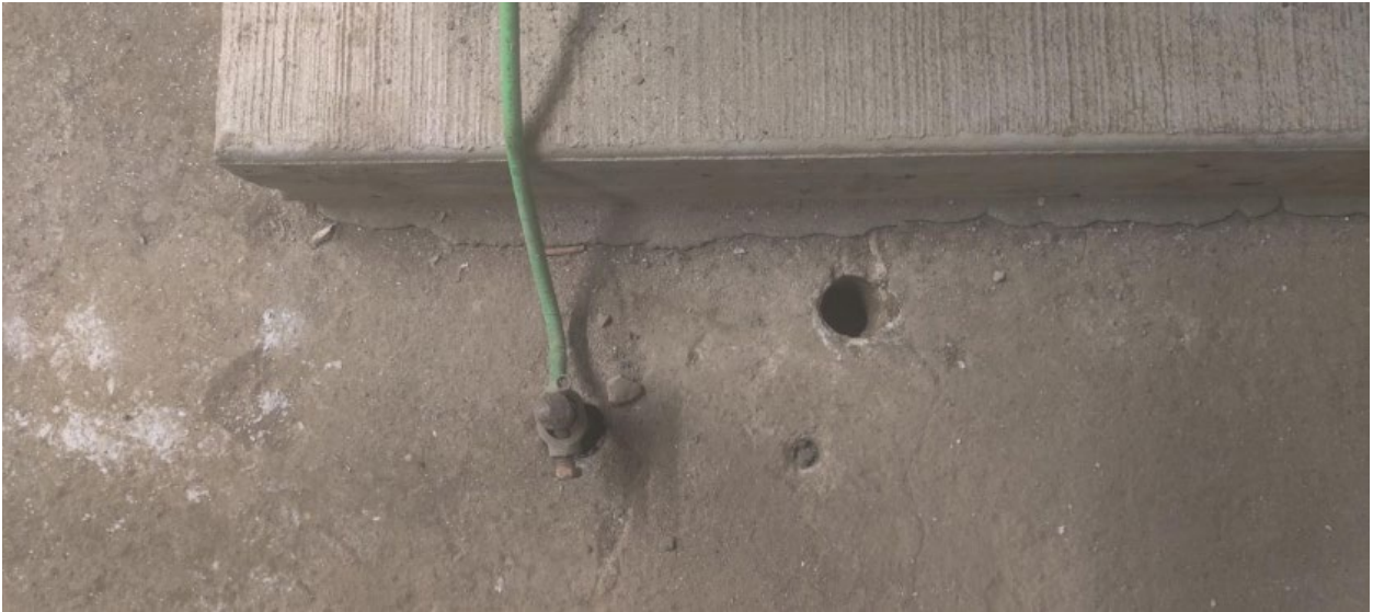
Photo 42 – Hole that needs to be sealed
