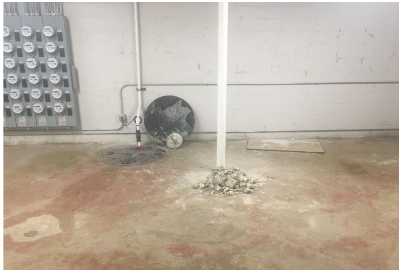
Photo 38 – Sump crock needs to be sealed permanently
