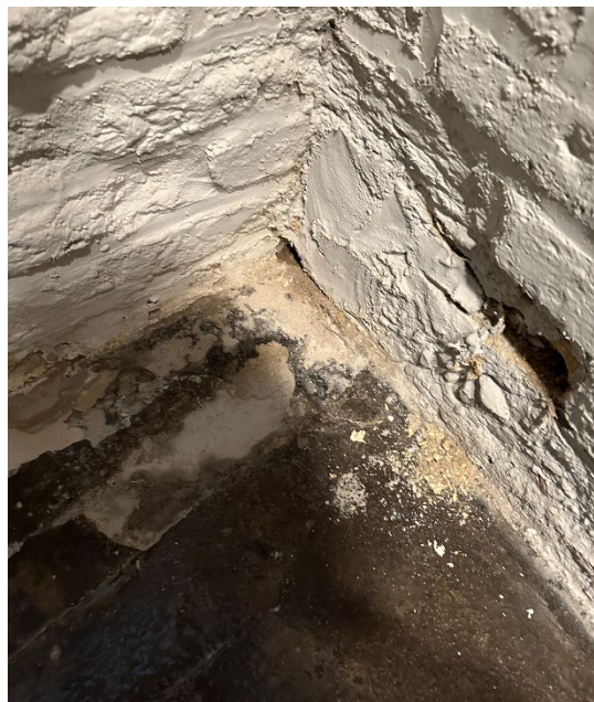
Photo 11 – Hole in masonry wall and slab
