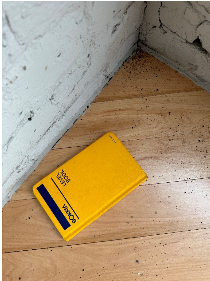
Photo 28 – Gaps between masonry wall and floor, cracks in the brick
