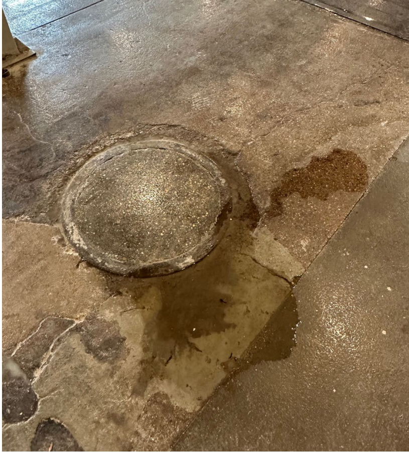
Photo 35 – Water intrusion at abandoned manhole
