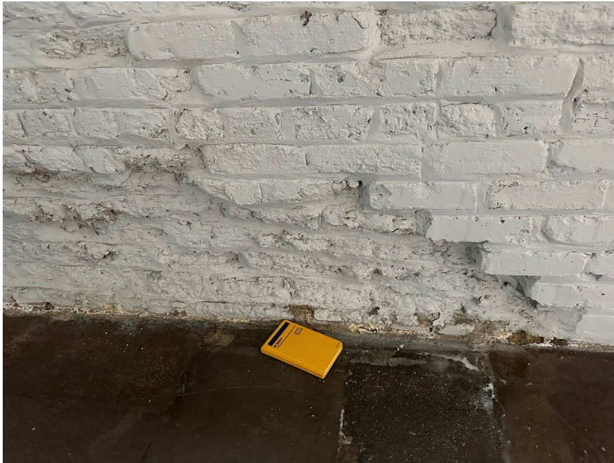
Photo 3 - Deterioration of masonry wall and gaps between the concrete slab and wall
