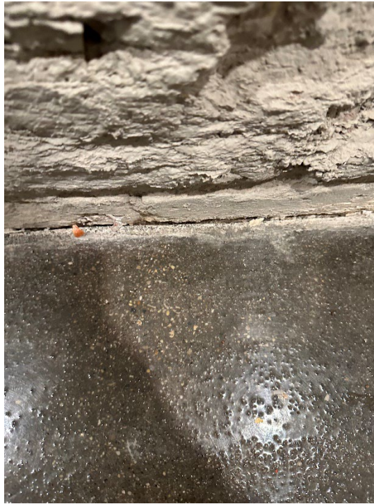
Photo 31 - Southwest hallway has gaps and holes all along the wall.
