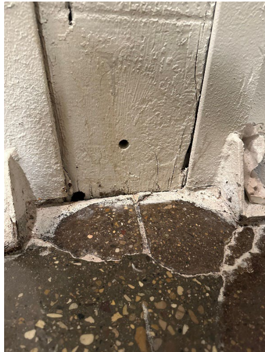
Photo 16 - Hole in the bottom corner of wood post
