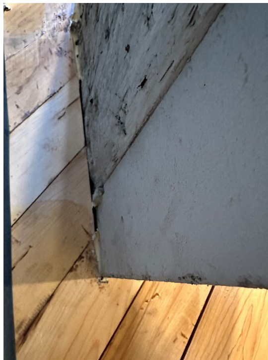
Photo 18 - Posts are not sealed all the way around and the wood beams are very porous
