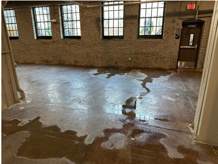
Photo 33 - SE corner near offices shows water getting in
