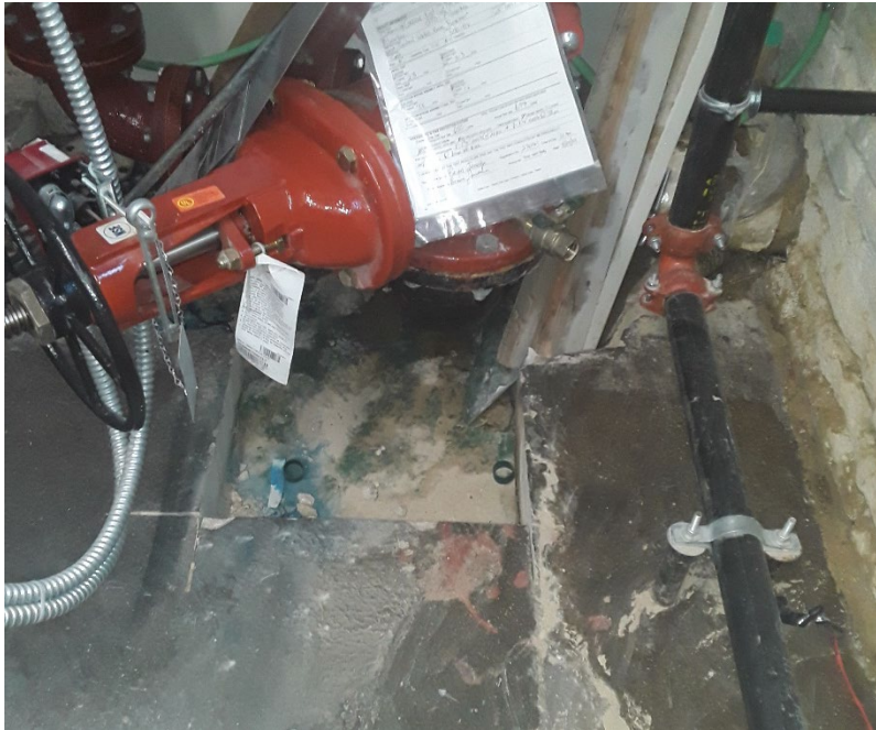
Photo 40 – Cut Slab that needs to be sealed
