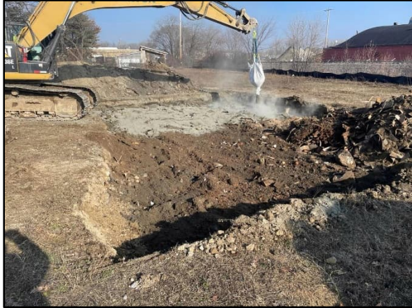
Photograph of stabilization activities for elevated lead detected in the soil. Photograph facing northeast.
