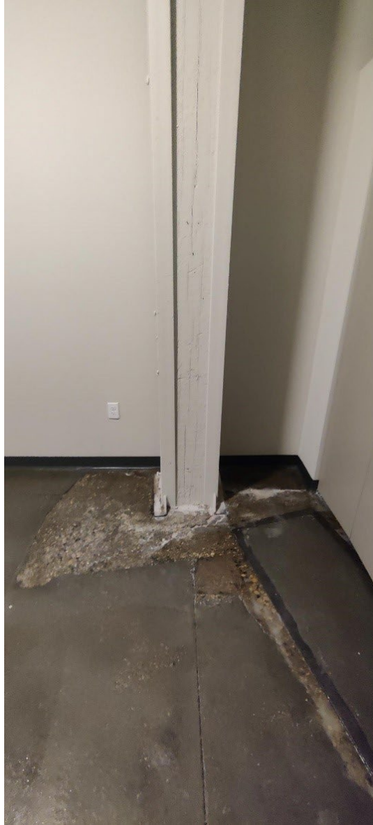
Photo 8: Unit 1036 - Wooden Pillar and cracks in bedroom 1
