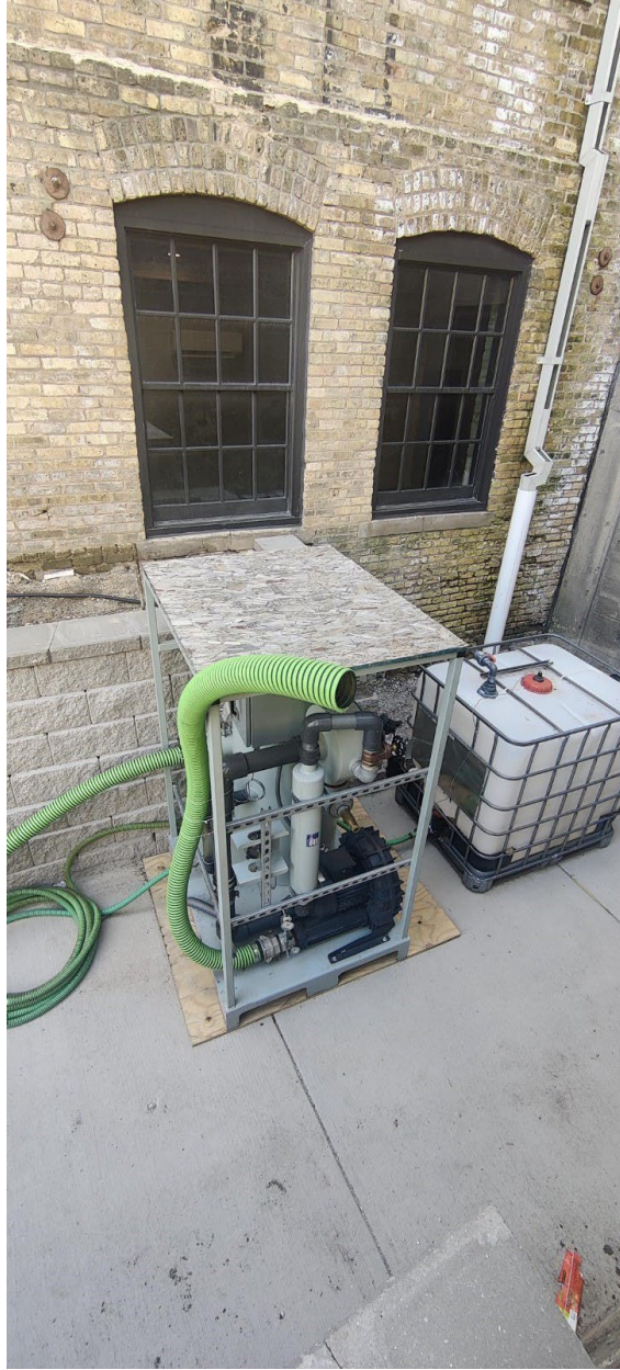
Photo 4: South 7.5 HP Blower Exhaust
