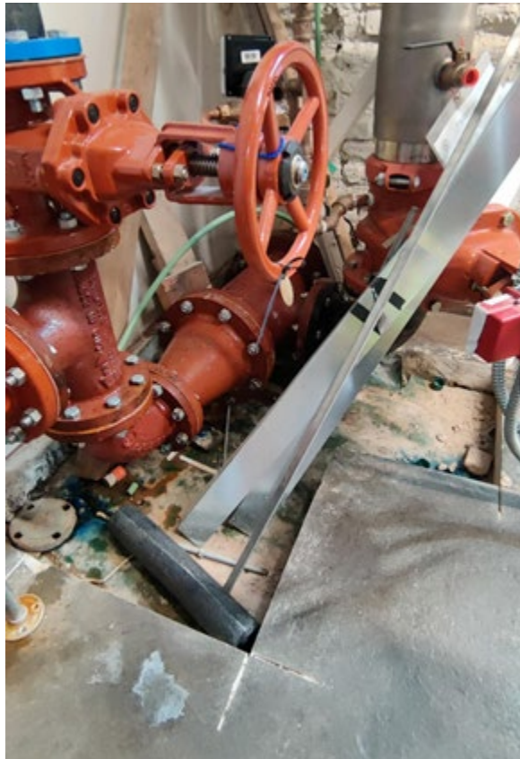
Photo 12: Unit 1052 – Open concrete area, exposed
