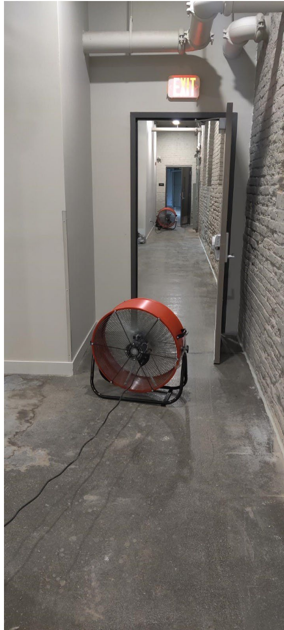
Photo 1: Ventilation in 1st Floor Hallway
