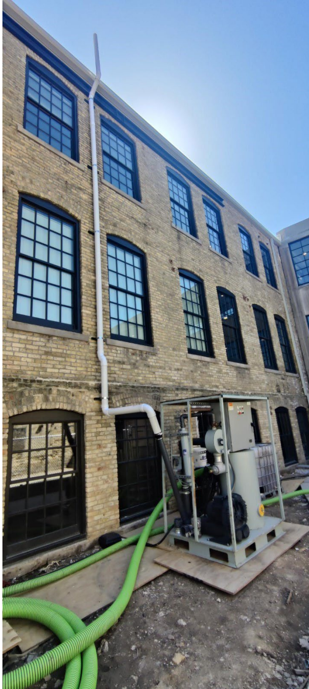
Photo 2: South 10 HP blower exhaust extended to above roof level
