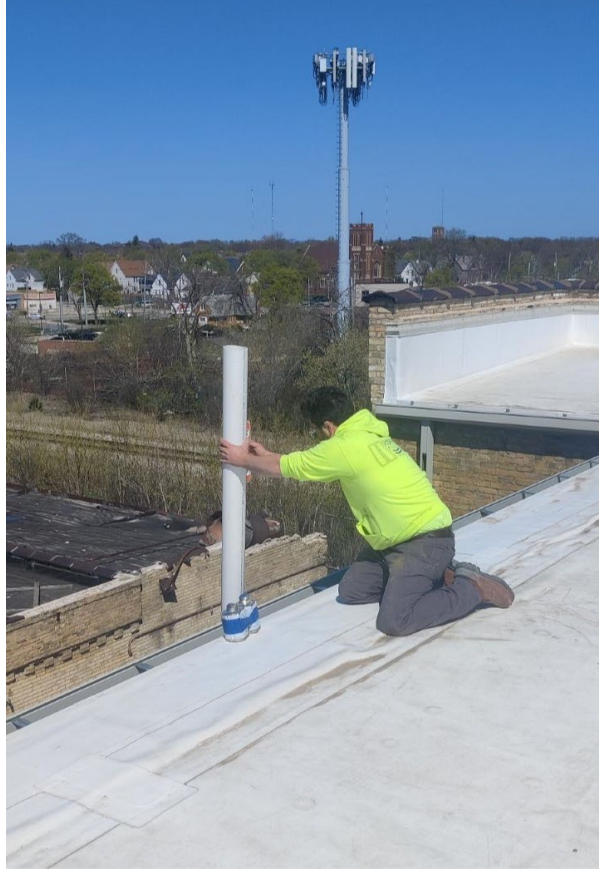
Photo 3: Unsafe sampling location – Needs U-pipe
