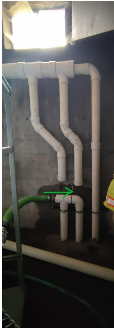
Photo 6: Water dripping from pipe in North Garage
