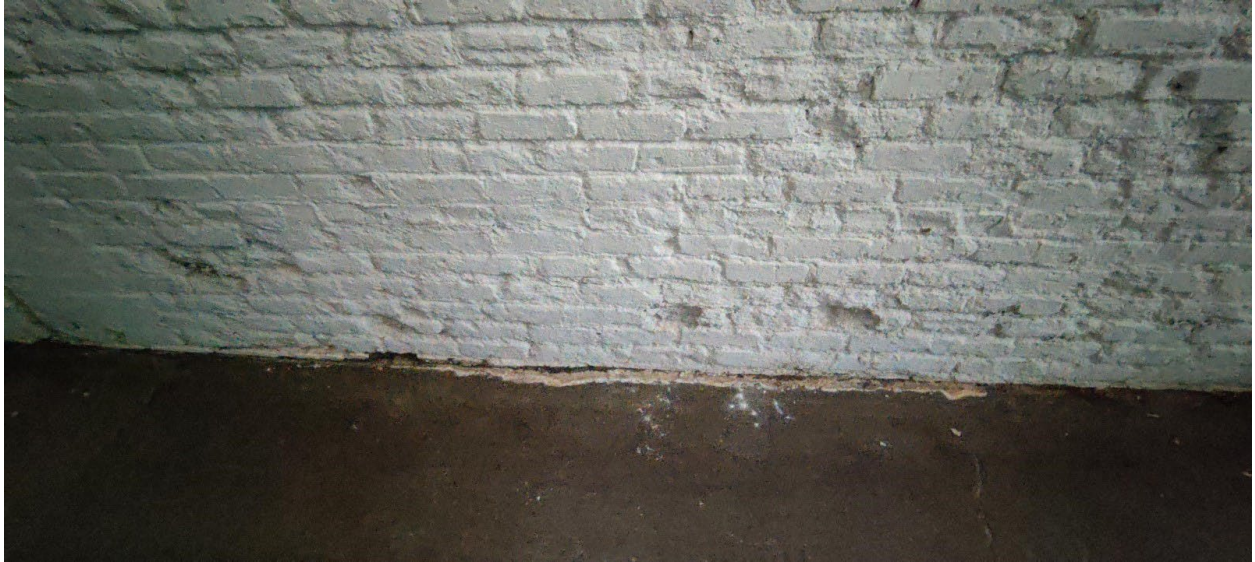
Photo 9: Unit 1039 – Cracks along the masonry wall
