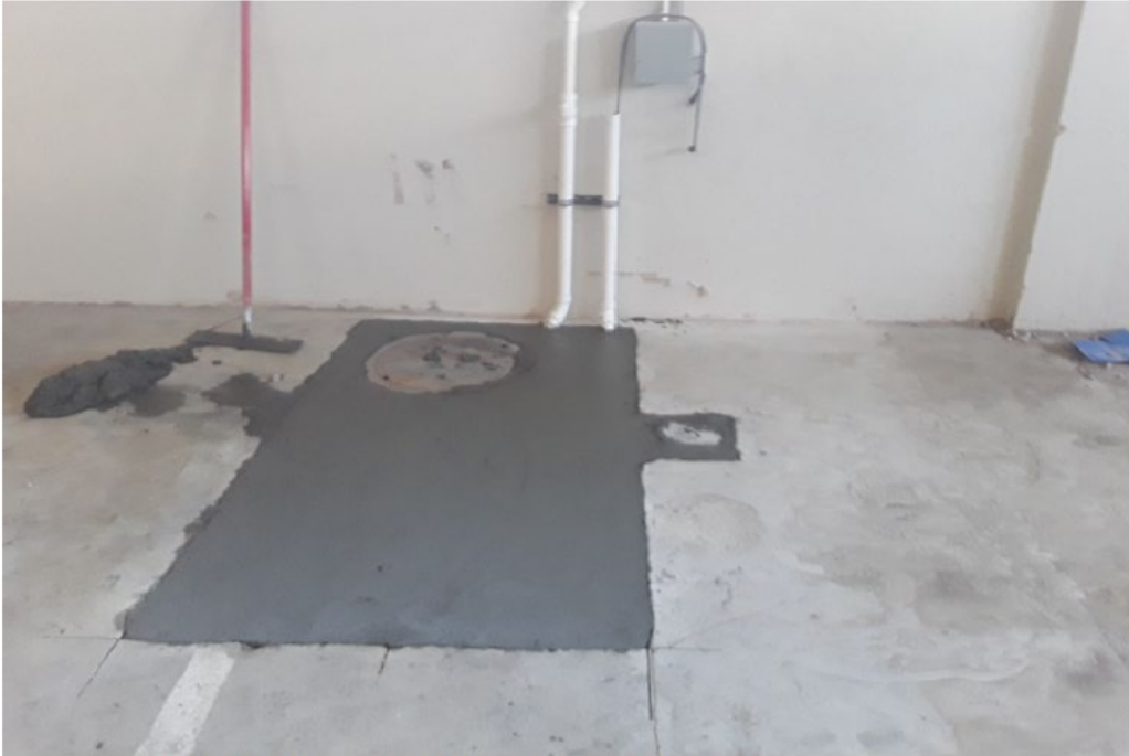
May 31, 2023 - Concrete Sealed Sump in Building 2A
