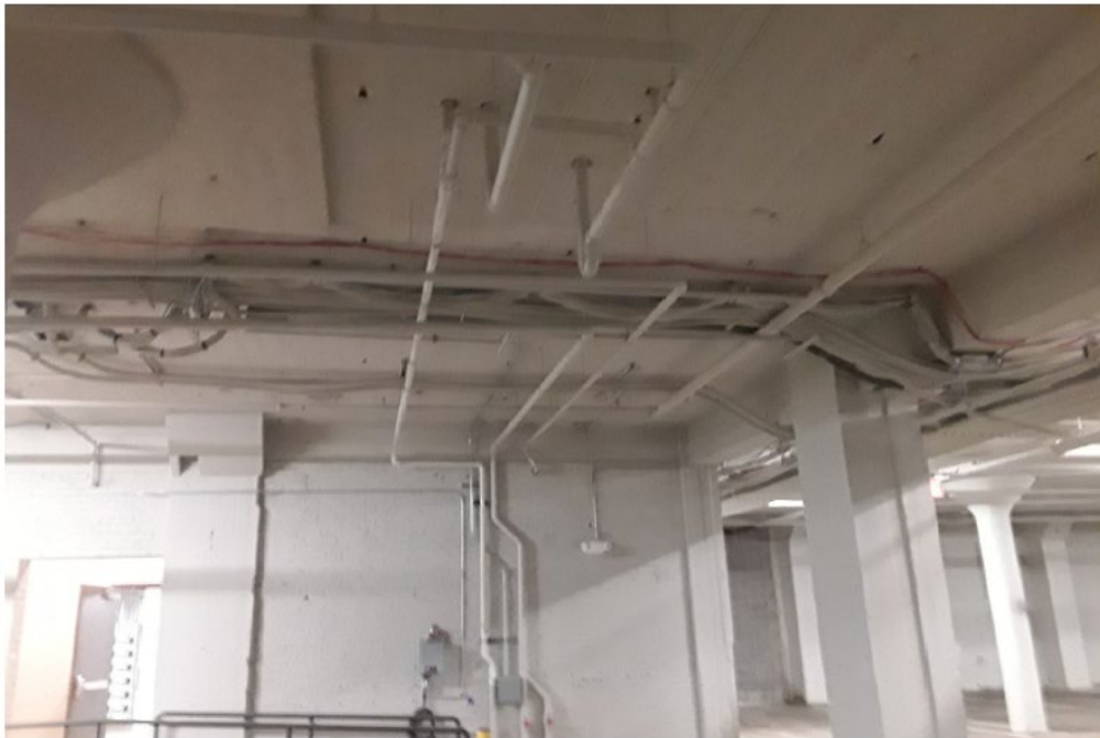
May 31, 2023 - Installed Discharge Plumbing to Overhead Storm Piping - Elevator Sump - Bldg 2A
