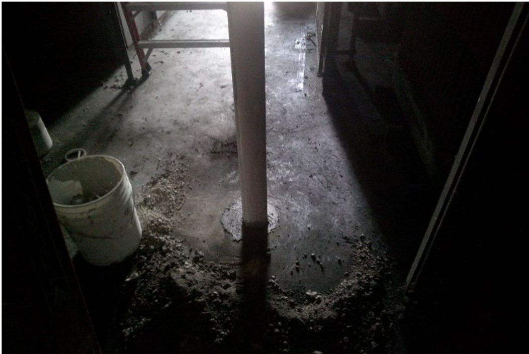
June 2, 2023 - Power House Sealed Vapor Extraction Point
