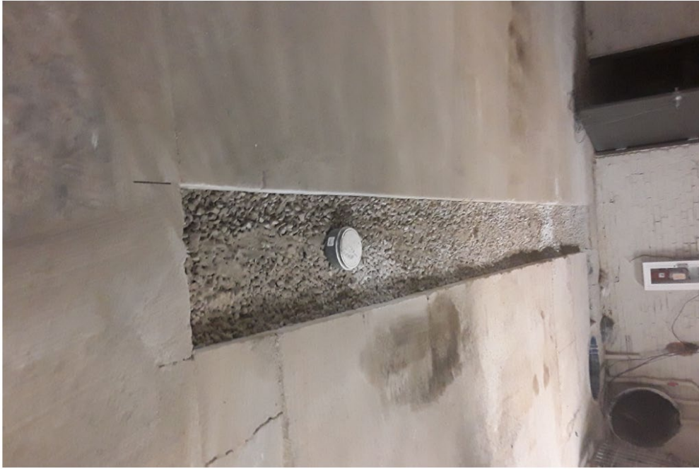
May 30, 2023 - Drain Tile and Inspection Port Ready for Vapor Barrier and Concrete at Building 1B-NE Elevator Pit Sump
