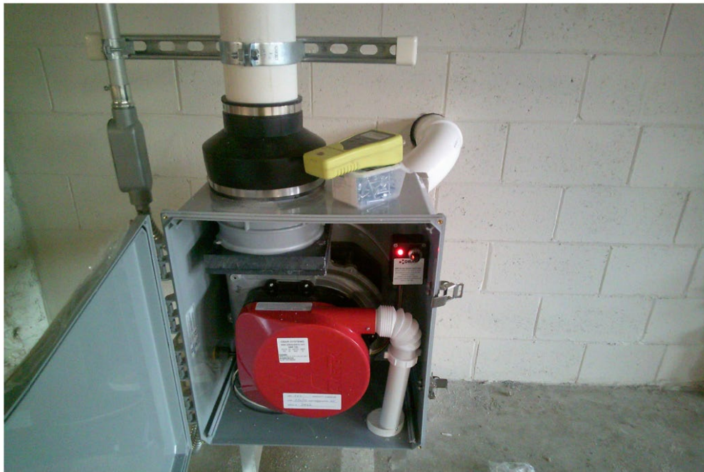
June 6, 2023 - Obar Fan with Active Electrical Connection
