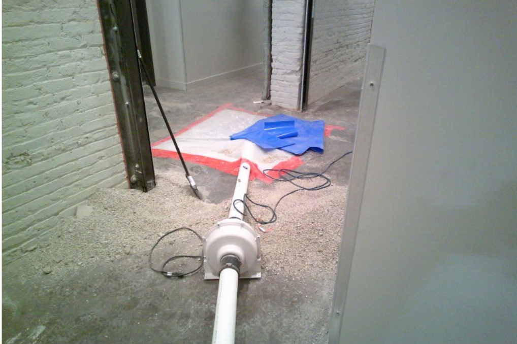
June 8, 2023 - GP501C Radon Fan Set Up at Access Point 1
