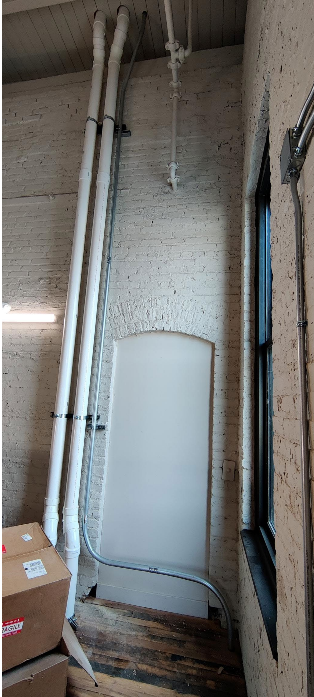
Picture 5 - Plumbing and electrical for Access Points 1 and 4 going up to the roof
