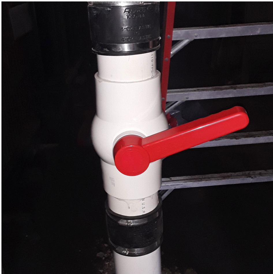
Picture 2 – Valve Connection in Powerhouse
