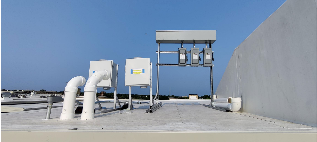
Picture 6 – GBR 89 Blowers on the Roof that are connected to Access Points 1 and 4
