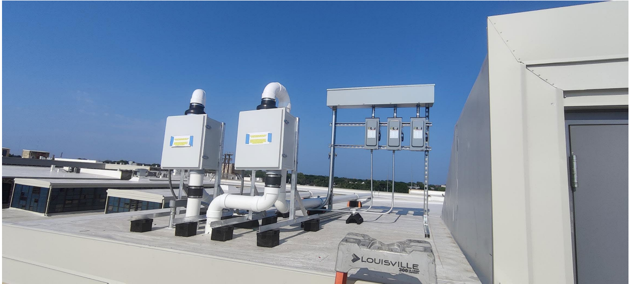
Picture 1 – Operation of Blowers 6 and 7
