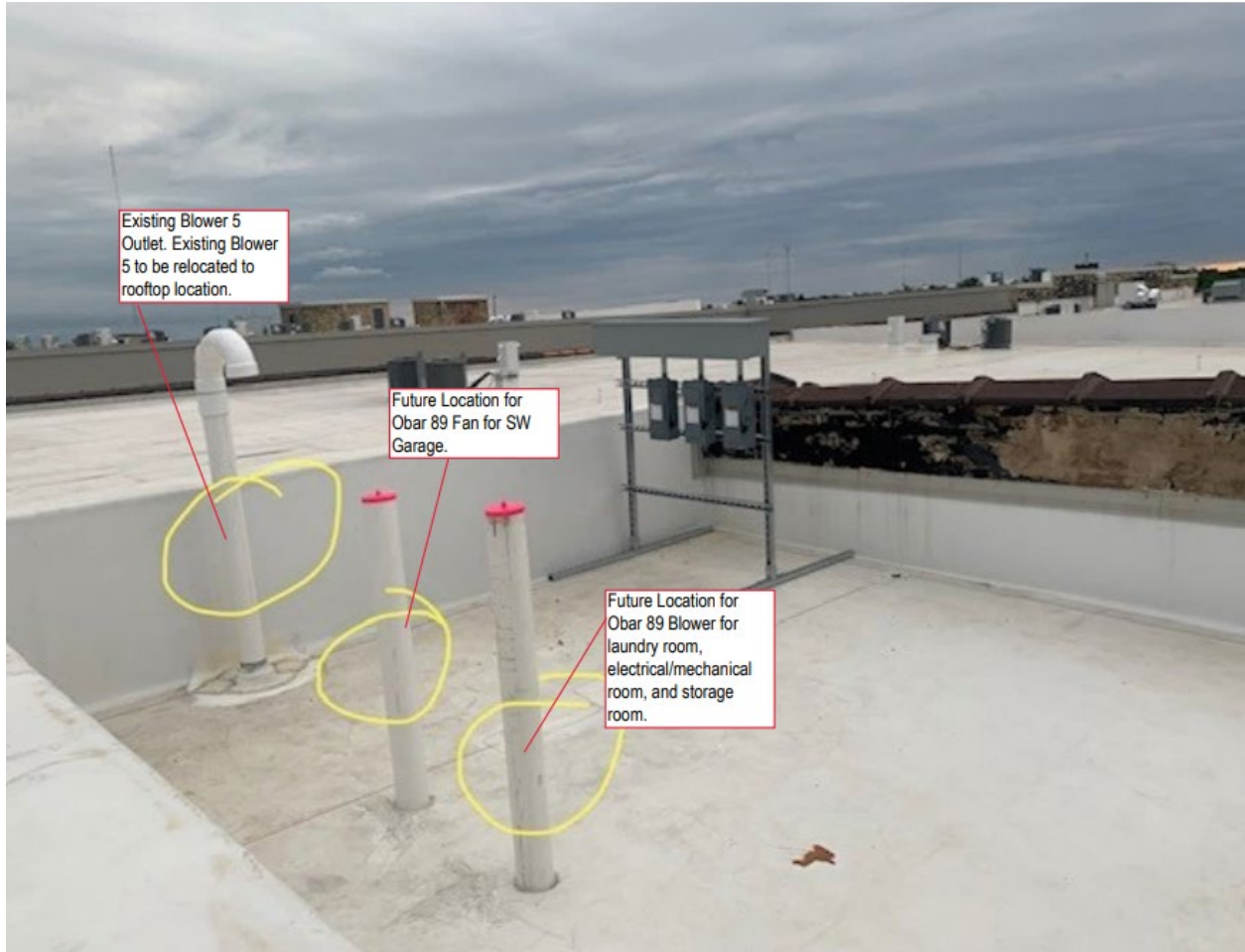
Picture 8: Ongoing installation of Blowers 10 and 11 on the roof above SW Garage
