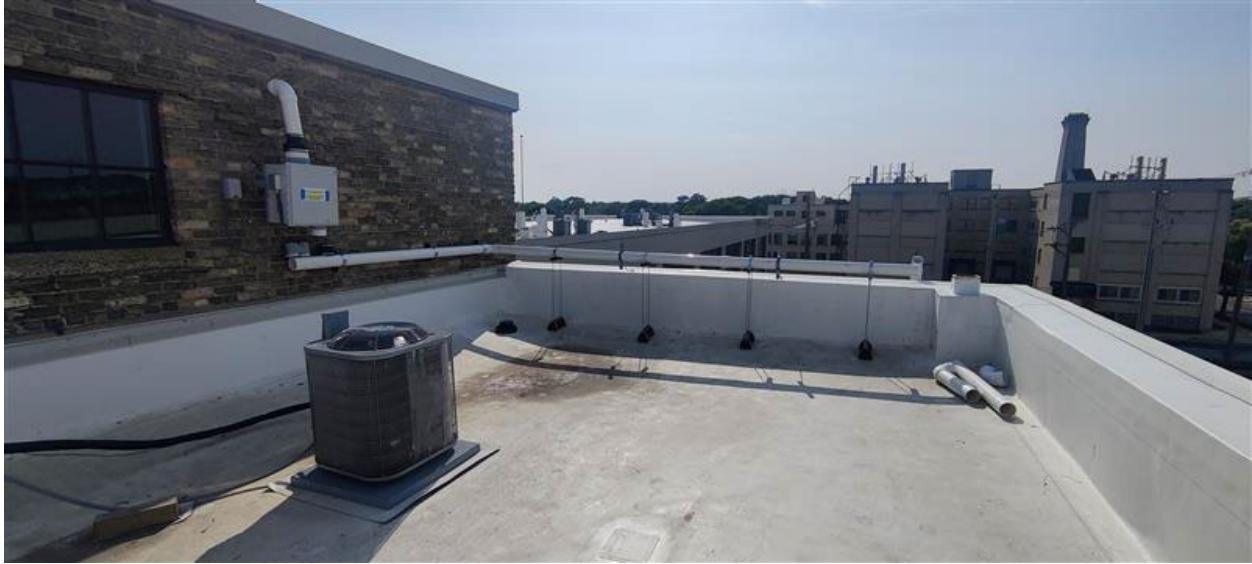
Picture 6: Ongoing installation of Blower 8 on the roof above N Mechanical room
