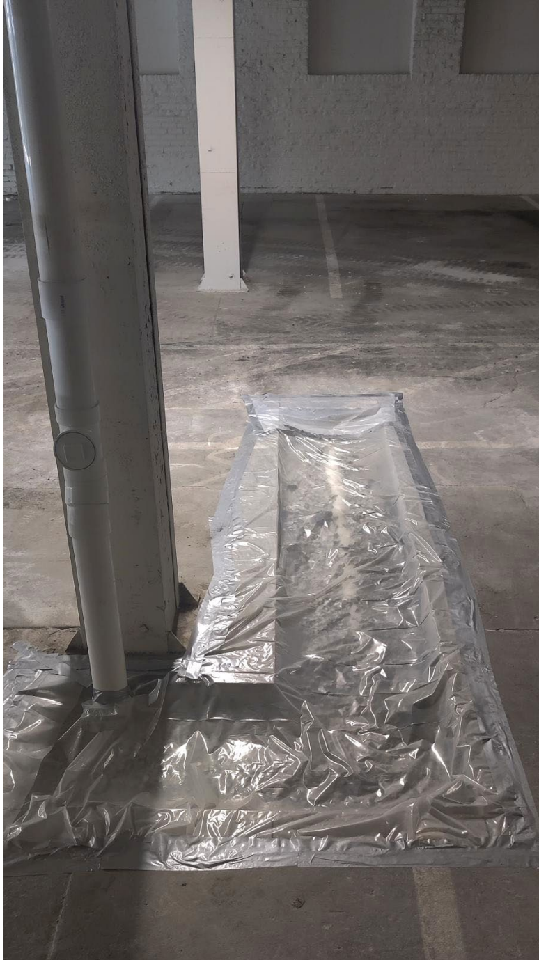
Picture 3: Concrete cut and removed from SW Garage area for the addition of access point for the Blower 11
