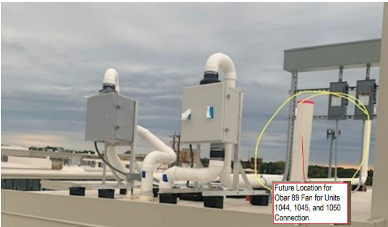
Picture 7: Ongoing installation of Blower 9 on the roof next to Blowers 6 and 7
