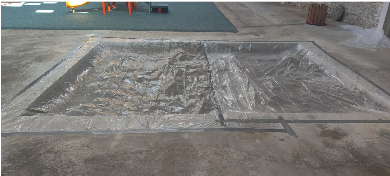
Picture 2: Concrete cut and removed from BB2 Pin Area in the Gym
