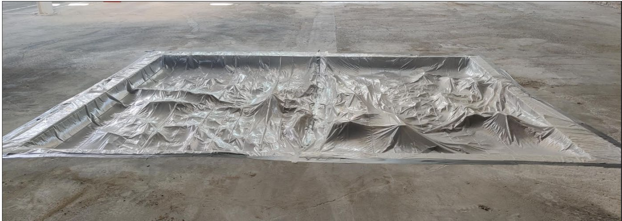
Picture 1: Concrete cut and removed from BB1 Pin Area in the Gym
