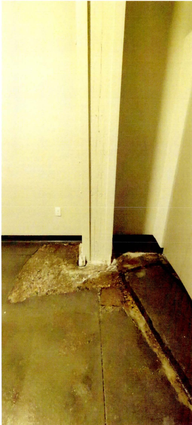
Picture 8: Unit 1036 - Wooden Pillar and cracks in bedroom 1
