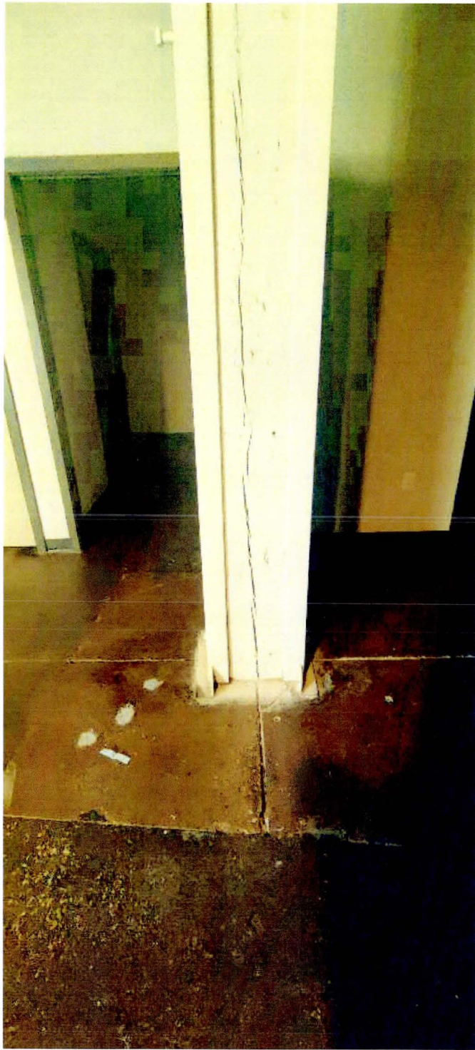
Picture 7: Unit 1026 - Wooden Pillar and cracks in the living room
