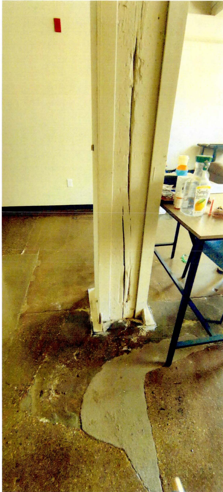
Picture 12: Unit 1040 – Cracks in wooden pillar and floor in living room
