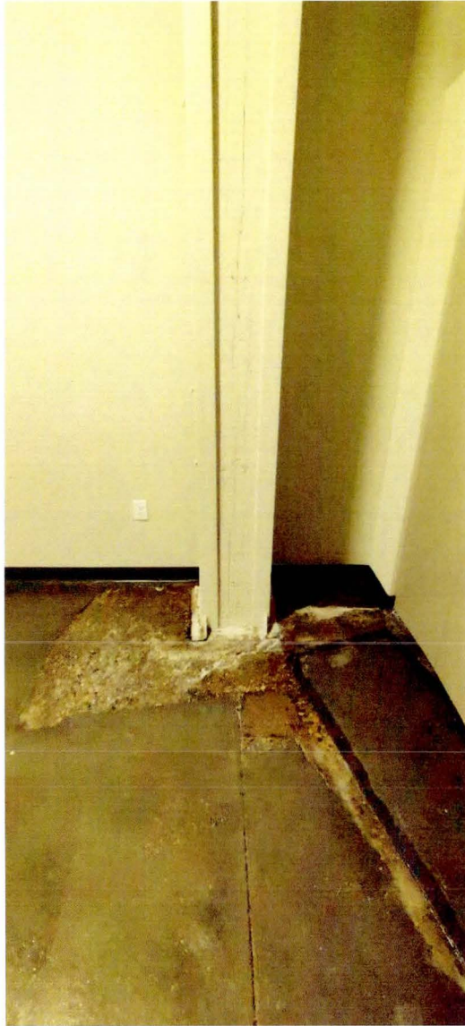
Picture 2: Unit 1036 - Wooden Pillar and cracks in bedroom 1
