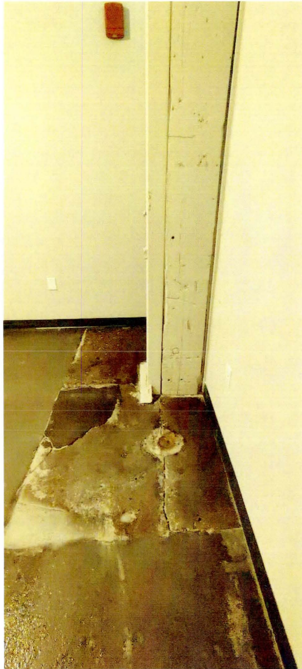
Picture 3: Unit 1025 - Wooden Pillar and cracks in the bedroom
