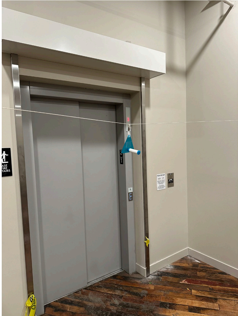
Picture 3 – Placement of Passive Sampler EB-02-A outside Elevator 1 on 2 nd Floor
