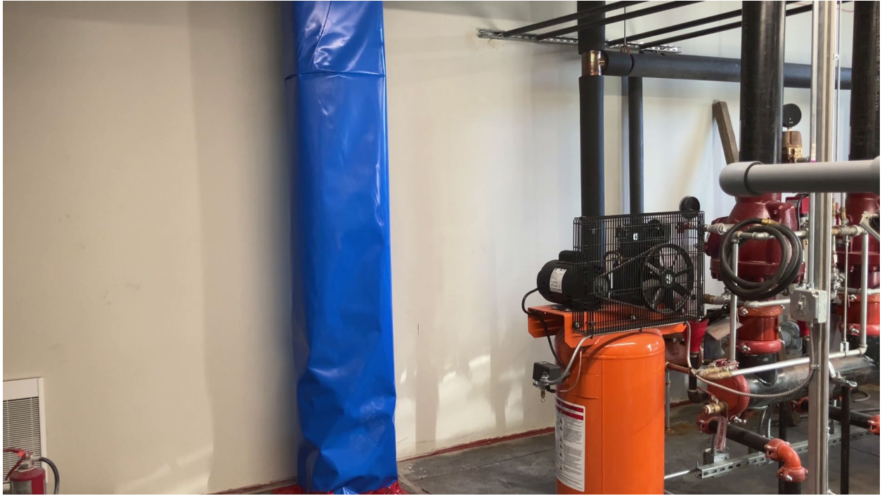
Picture 3. Vapor Barrier Sealed Column located in 1052 Mechanical Room
