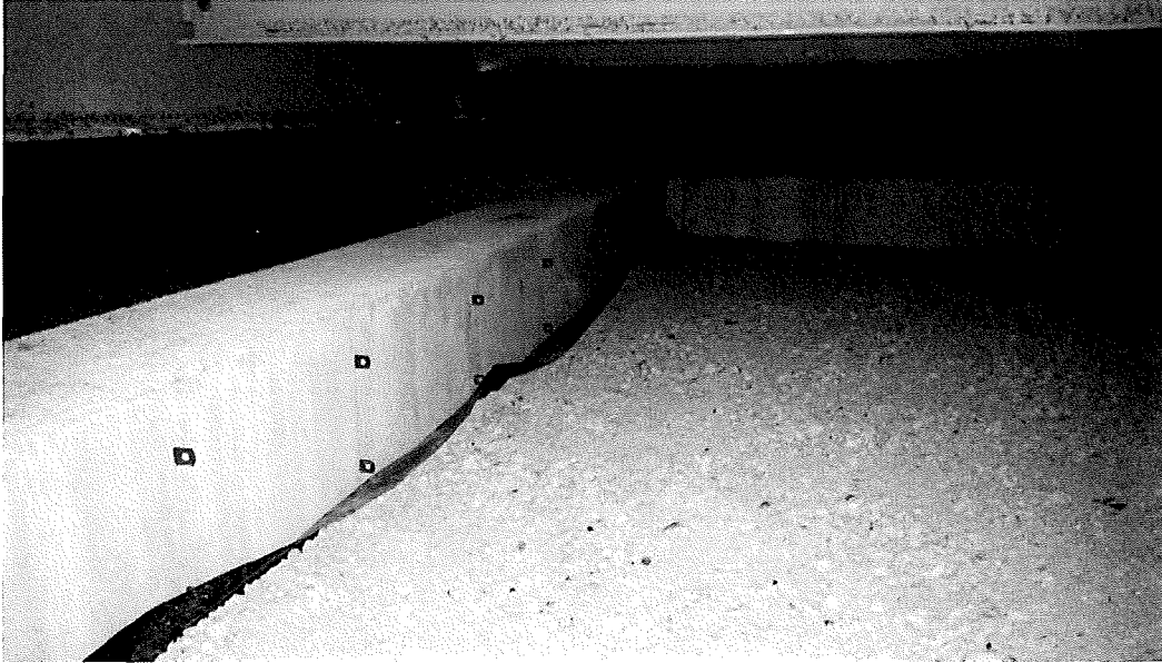
Photo 9: Typical crawl space area showing concrete grade-beam foundations, geo-membrane, and gravel base, approximately column EE14.
