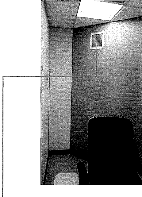
Photo 1: 1301 Canal; typical office area supply air duct, mezzanine level, column L2.5.
