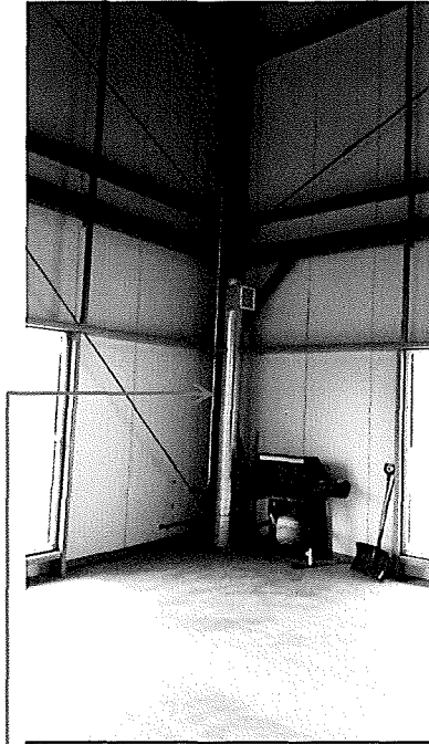
Photo 5: 1207 Canal; typical warehouse space supply air duct, column E17.
