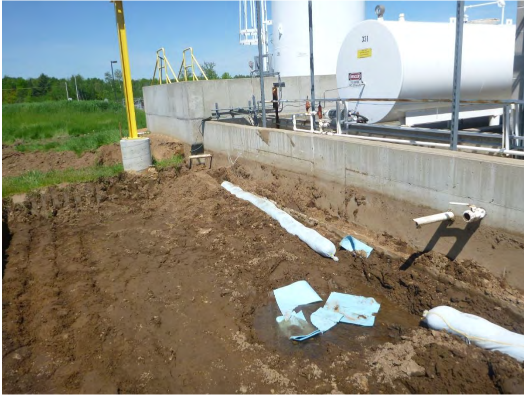
Point of spill, note secondary containment structure impedes further excavation.
