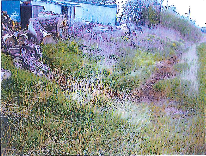
View to the southeast, west side of 8655 N. 43 rd Street. Shows flow of discharge from under the bark and debris to the west, and then southward along east side of ROW.
