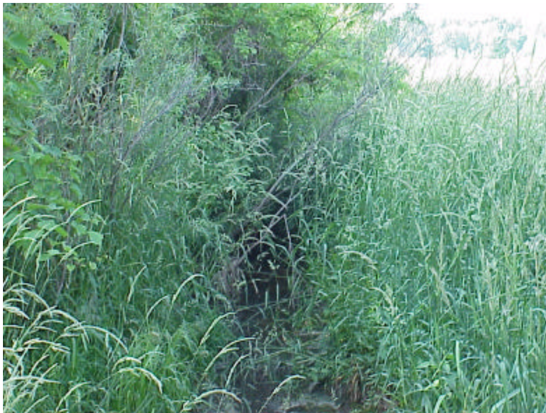
Figure 40. Thick, overhanging grass was common throughout the survey site on Larson Creek.
