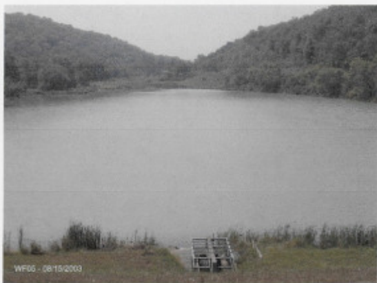
Figure 1. Seas Branch Pond from dam embankment looking upstream with outlet in foreground. (Vernon County Land & Water Conservation Department)
