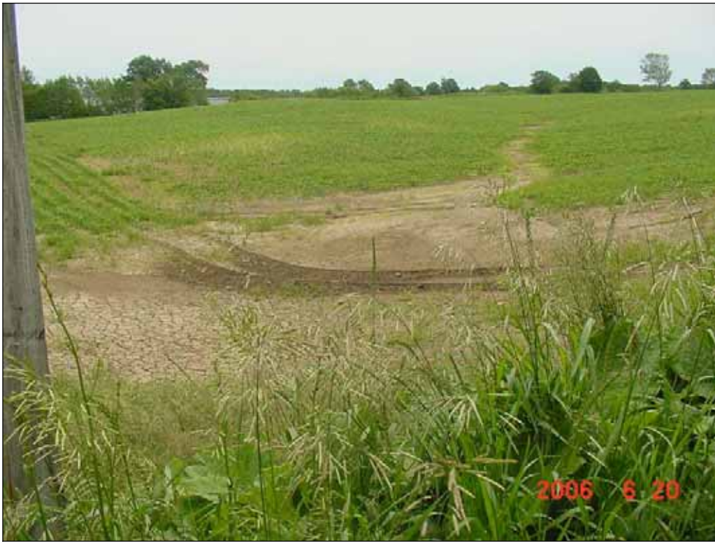
Site 6 - Eroded Corn Field at SE Corner of Racetrack Road and Hwy. JJ
