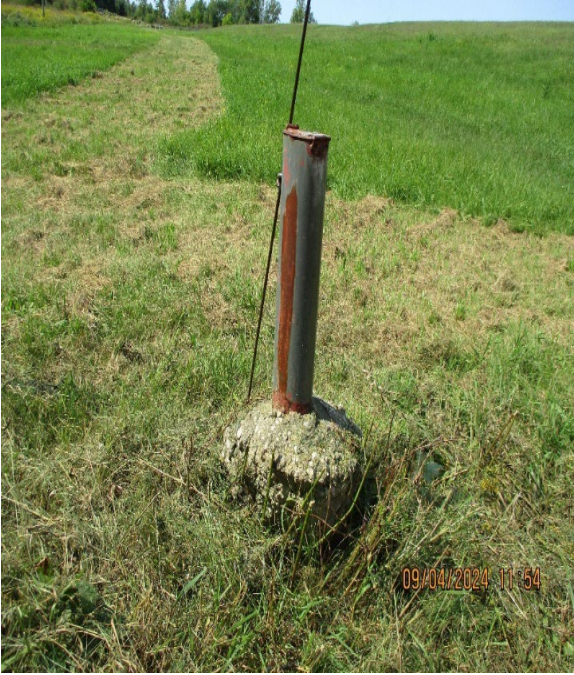
Photo 5: Groundwater monitoring well with concrete surface seal that has heaved out of the ground due to frost
