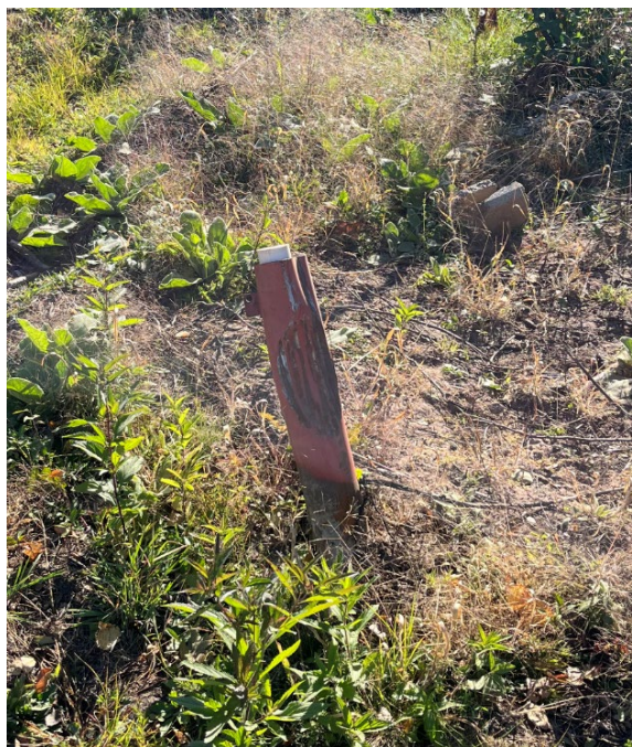
Photo 10: Damaged groundwater monitoring well that may need to be replaced.
