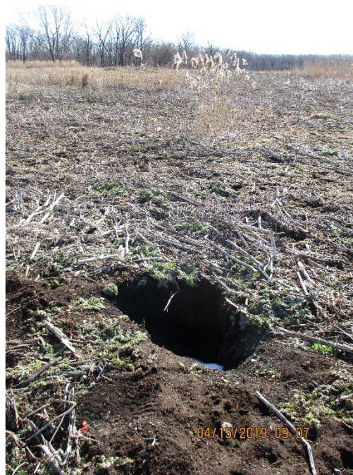
Photo 4: Animal borrow hole on landfill cover.
