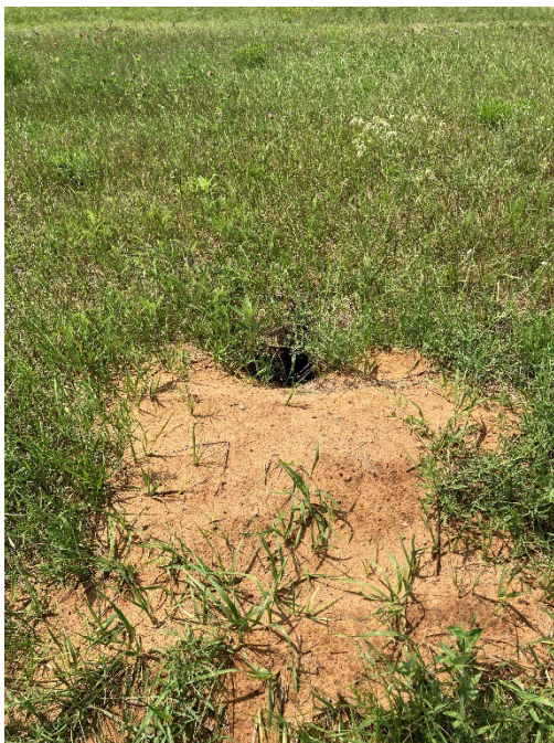
Photo 3: Animal borrow hole on landfill cover.3
