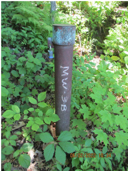
Photo 14: Groundwater monitoring well.
