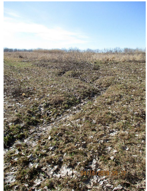
Photo 1: Gully type erosion on landfill cover.
