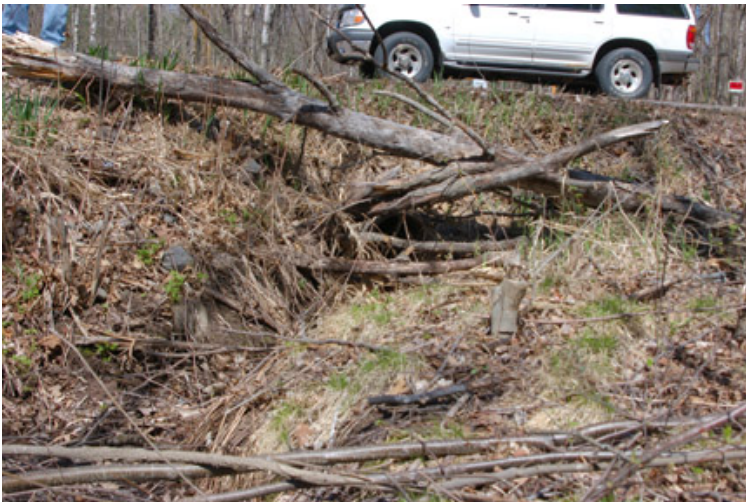
Eroded channel flows to the lake.
