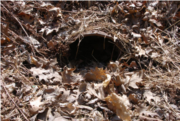
Culvert #7 w/sediment deposition is improperly sized.
