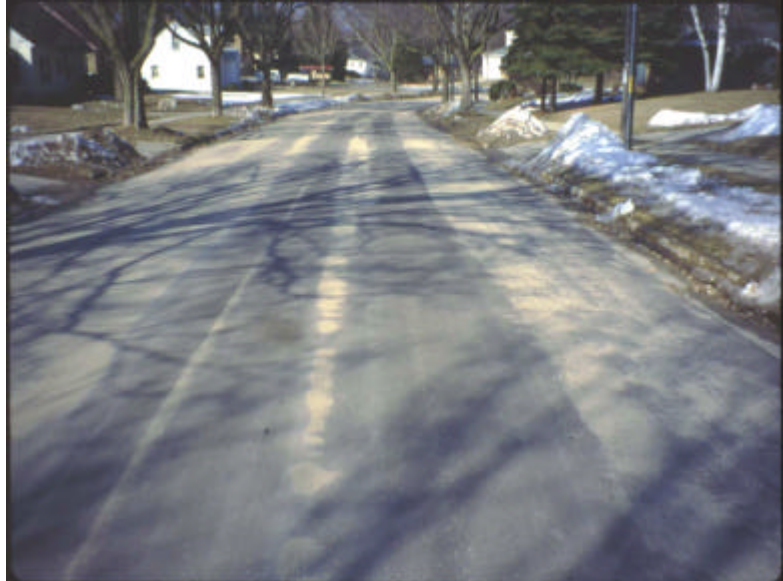
Road Salt and Sand Accumulation
